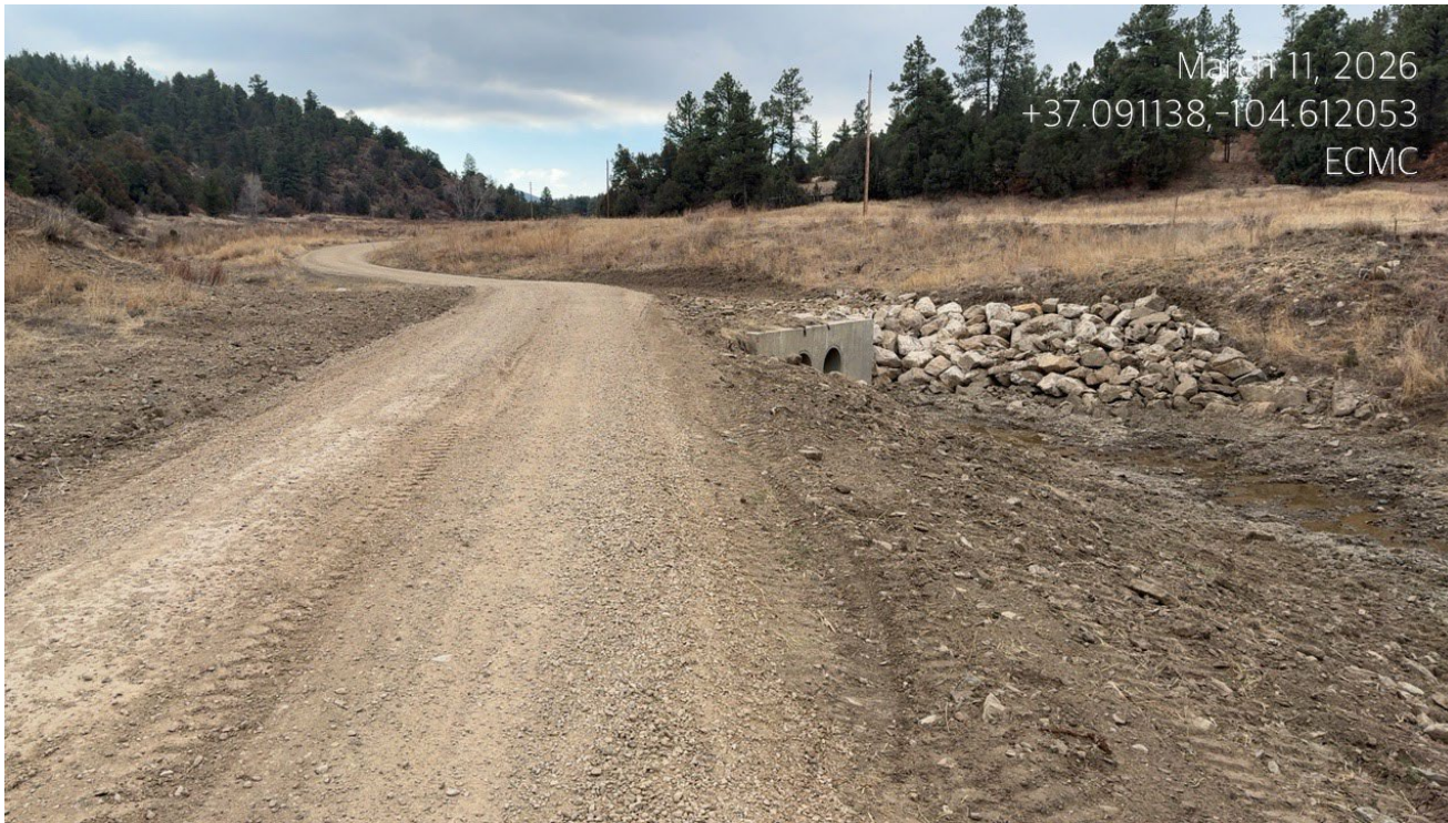
Photo 1. Facing southeast along the access road. Additional BMP's appear to have recently been installed.
