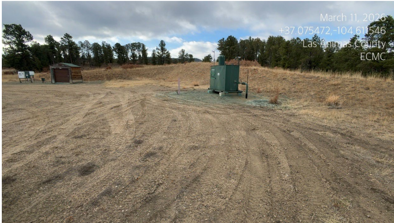
Photo 4. The vegetation around the equipment has had recent herbicide treatment.
