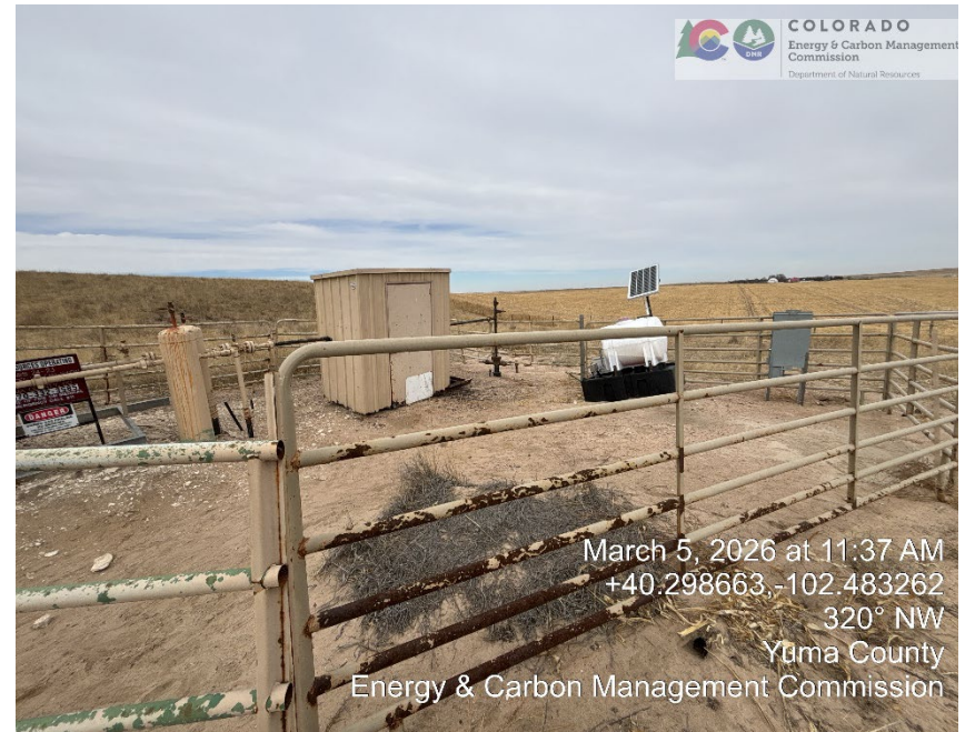
VGS, VGS Shed, Wellhead, Chemical drum, and Electrical panel
