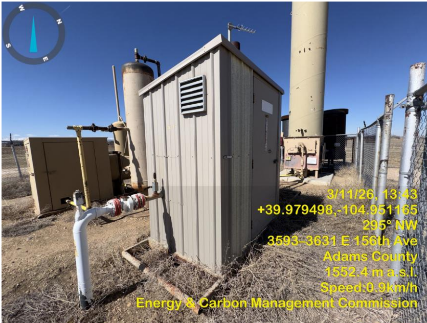
Photo 13 Gas meter Run.
