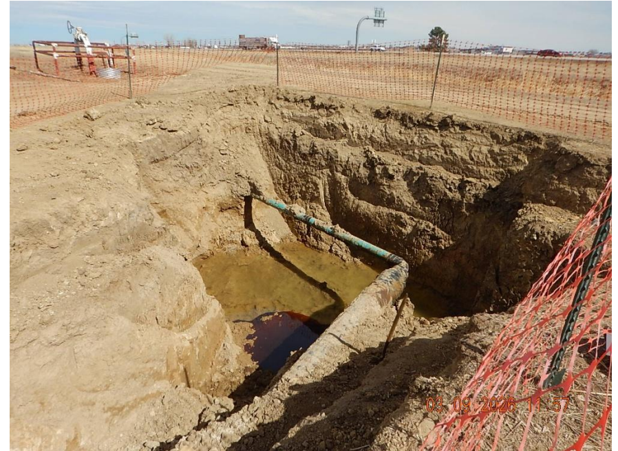
View into excavation of large off location flowline measuring approximately 20" in diameter transitioning down to 6" diameter flowline via welded pipe reducer. This flowline is not the reported source of the release. Free oil product is seen floating on the surface of ground water in excavation.
