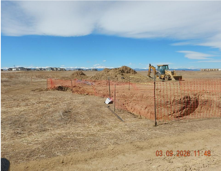
View looking west of fenced excavation at KPK Facility S4BW spill/ release. Spill Id # 493326 @ 40.098305, -104.981653
