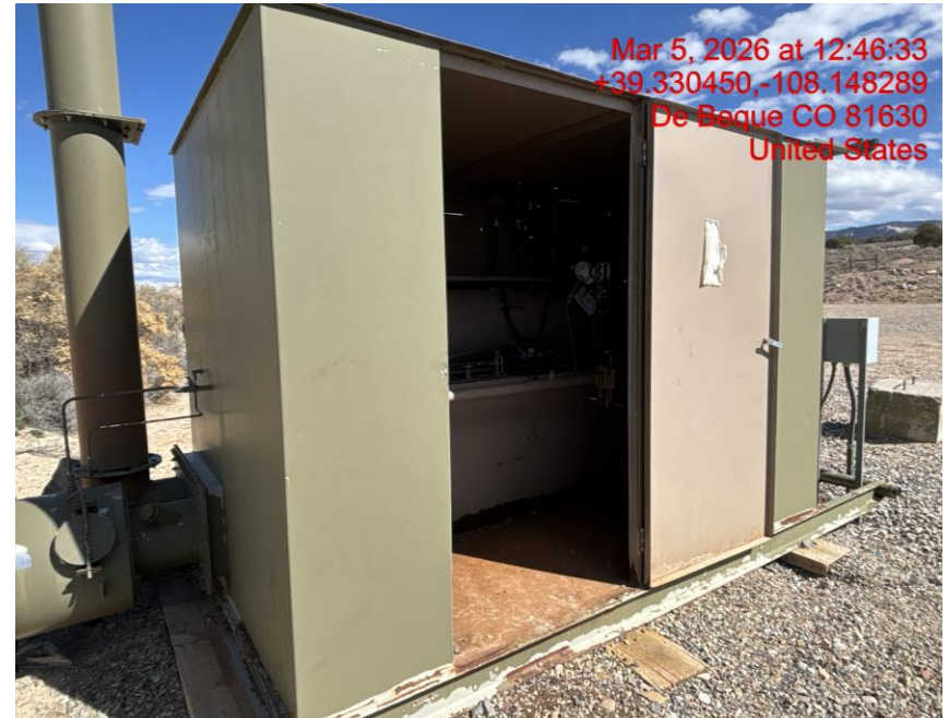
Unsecured Separator Door – Photo #02981
