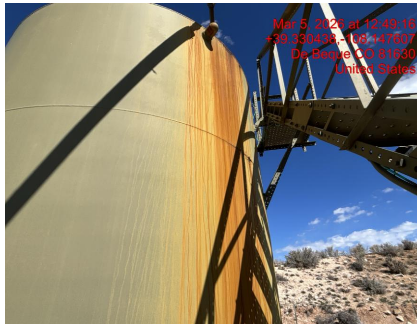
Tank Corrosion/Staining – Photo #02986
