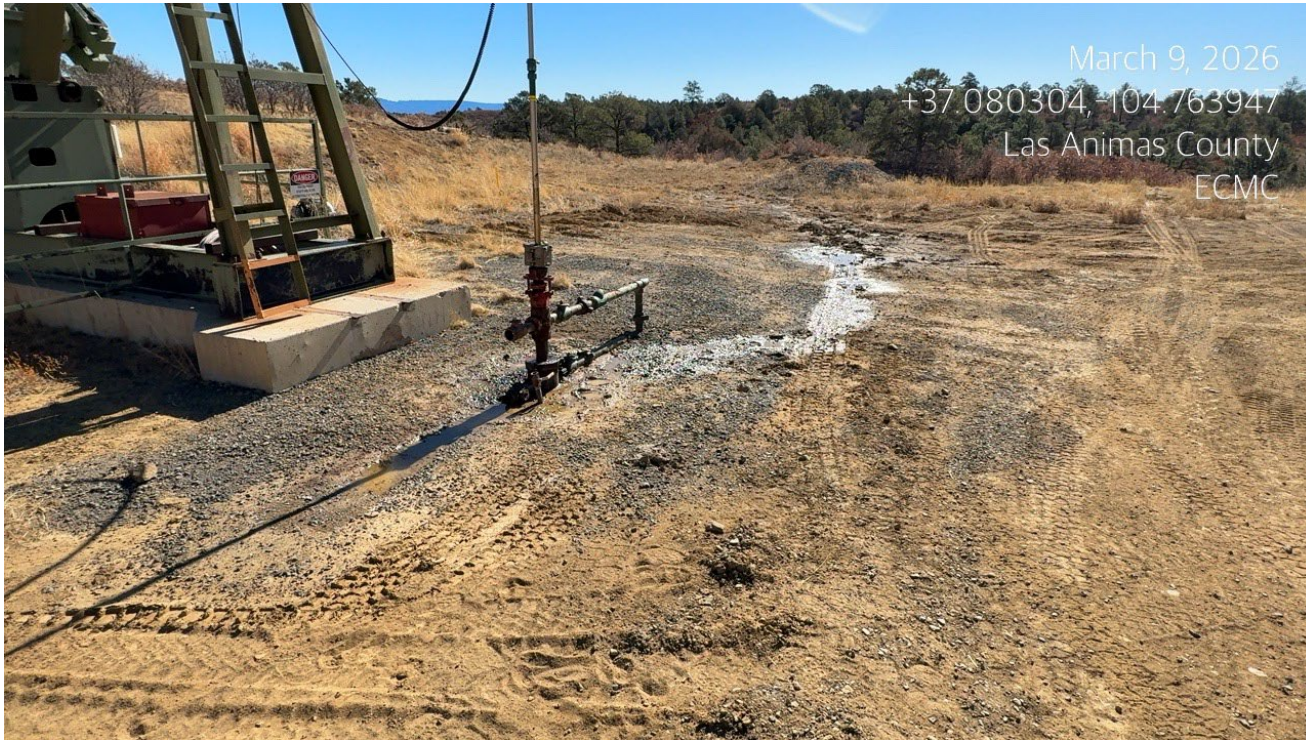
Photo 2. There was a dripping leak at the wellhead.
