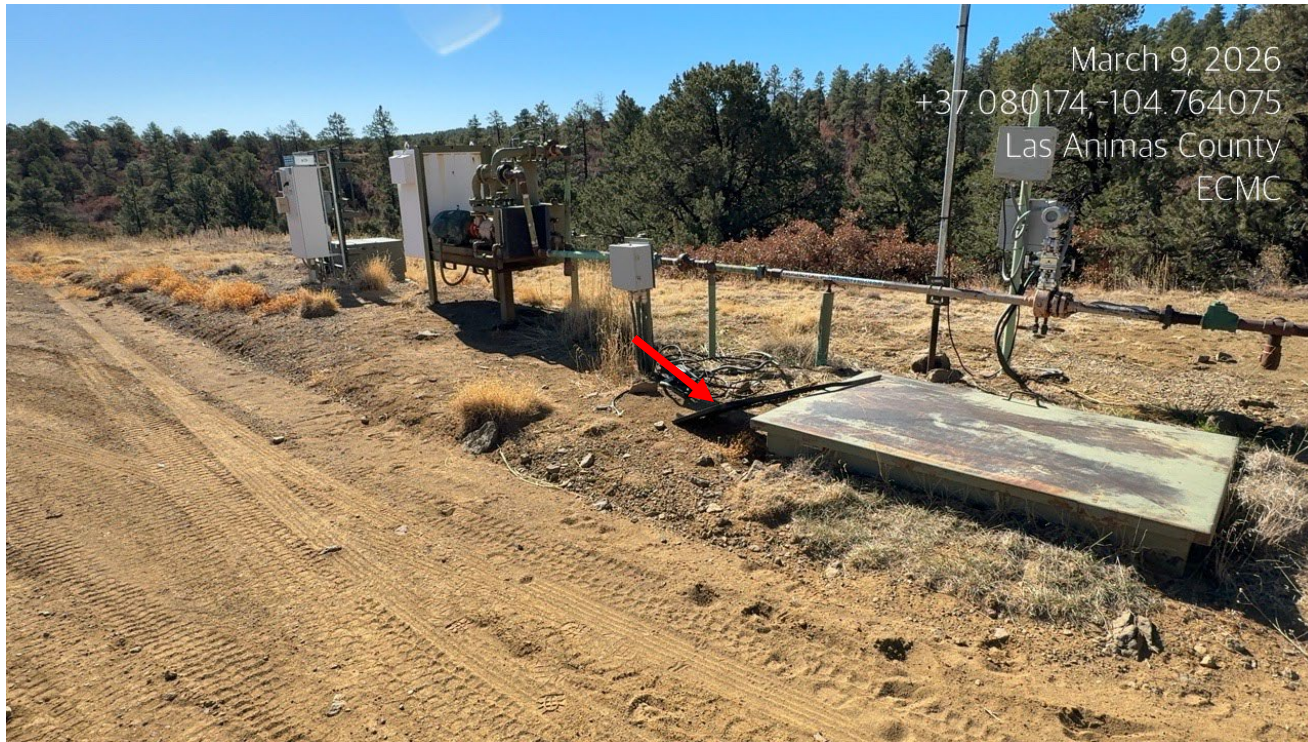
Photo 3. The well sign has fallen over and needs to be reinstalled.
