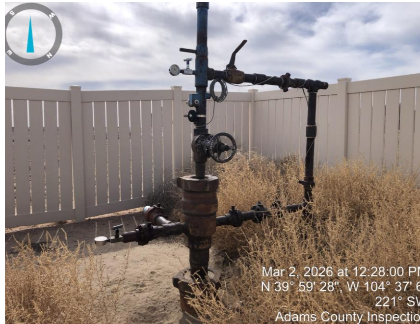
Photo #3 Well head and weeds throughout location (in and out of berms).
