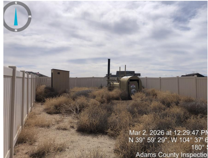
Photo #2 Meter & separator and weeds throughout location (in and out of berms).
