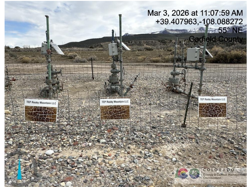
Photo # 4545 Wellhead signs damaged & illegible
