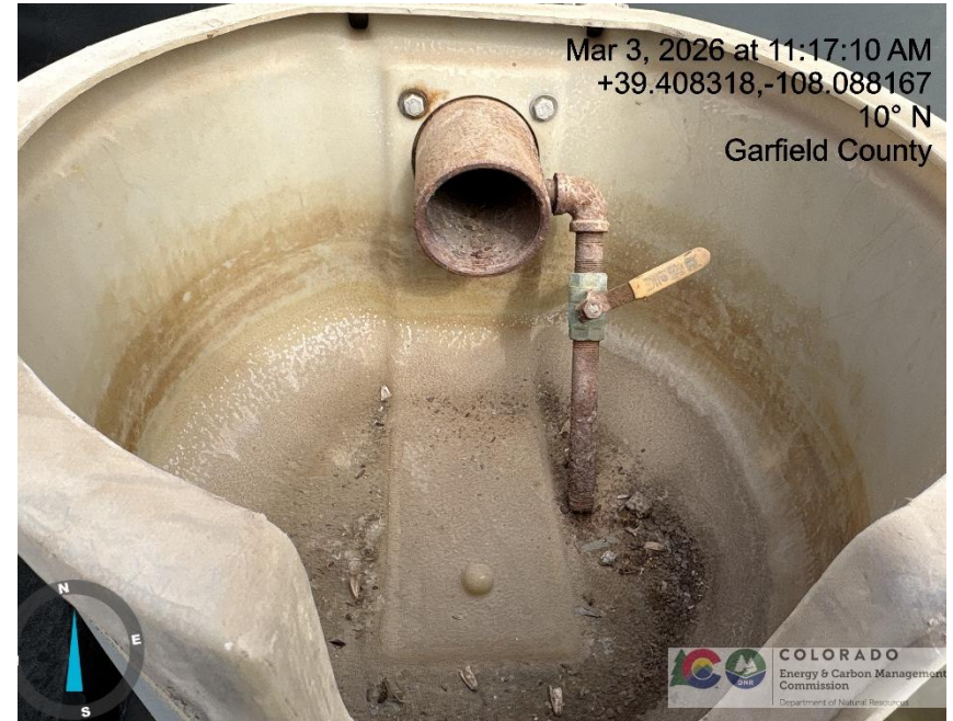
Photo # 4541 Open ended load line
