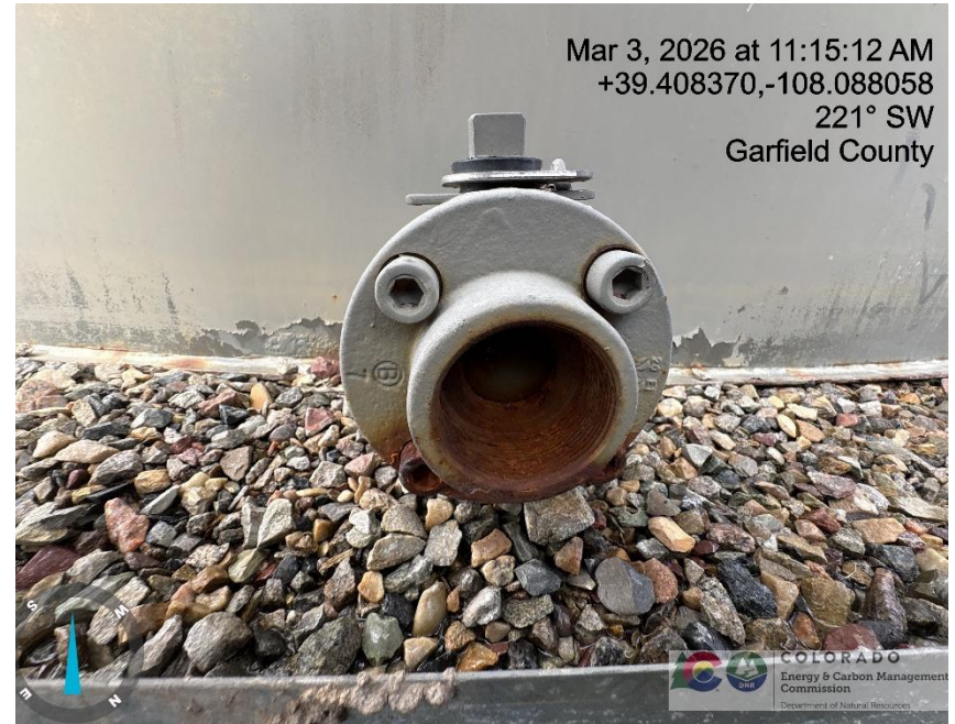
Photo # 4537 Open ended load line
