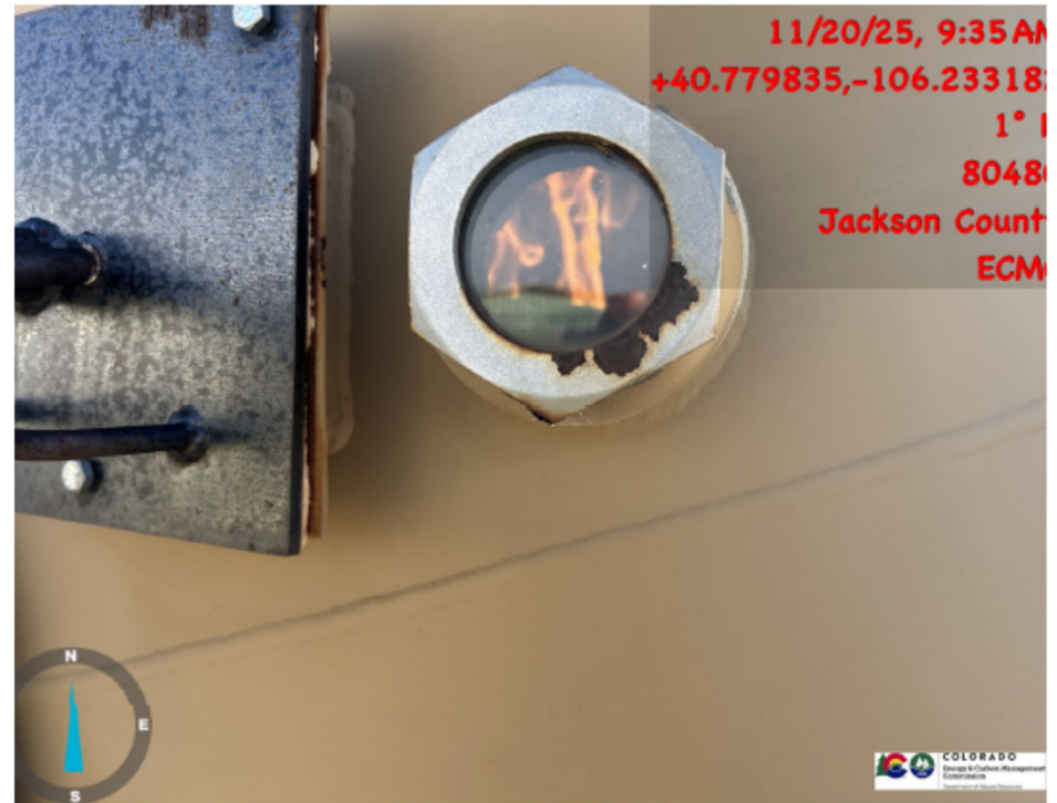
Previous inspection /audit photo of ECD running
