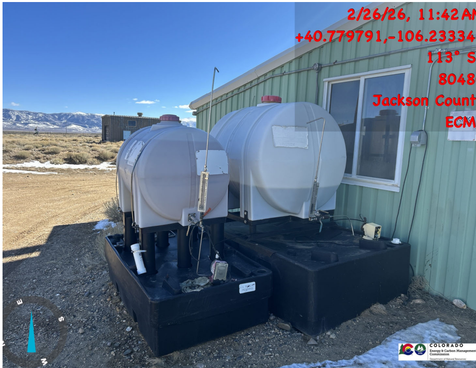
Recent inspection /audit of illegible tank labeling
