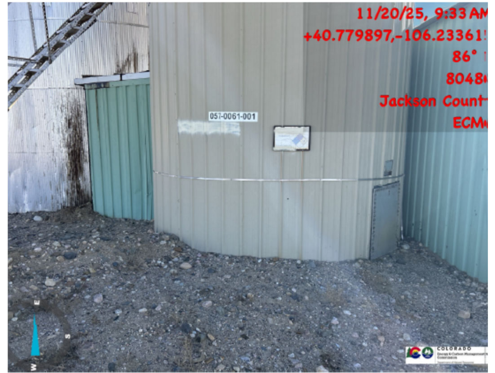
Previous inspection /audit of illegible tank labeling
