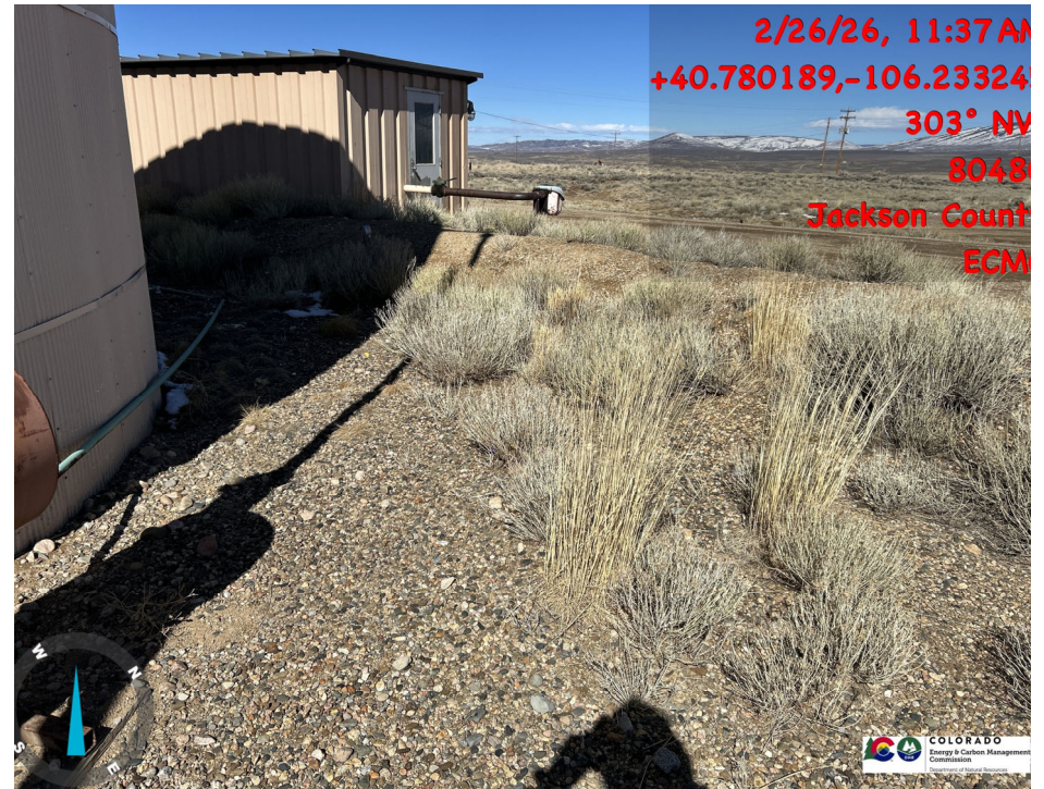
Weeds throughout secondary containment
