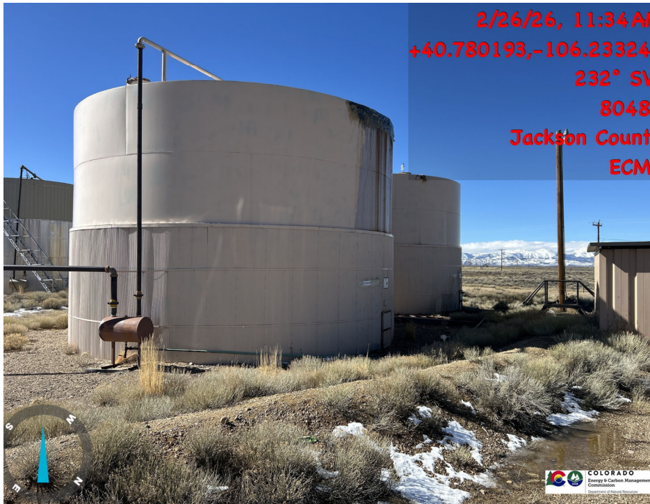
Recent inspection/audit of crude tanks and fiberglass patch
