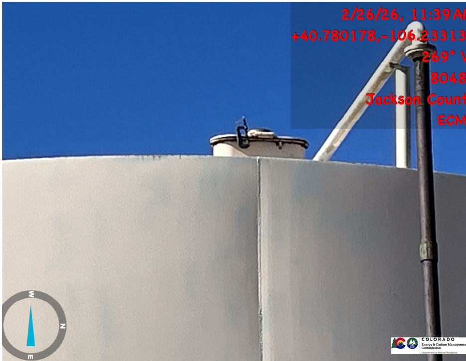
Recent inspection/audit of thief hatch being held shut with a C-clamp, lack of mechanical integrity.
