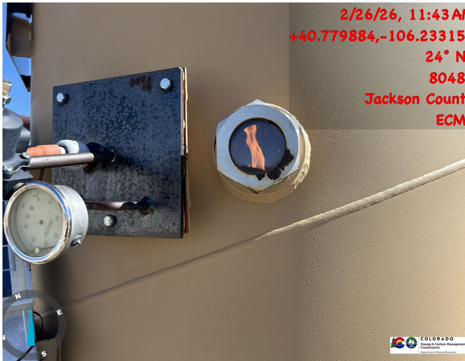
Recent inspection /audit photo of ECD running
