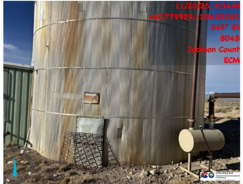
Previous inspection /audit of illegible tank labeling and debris
