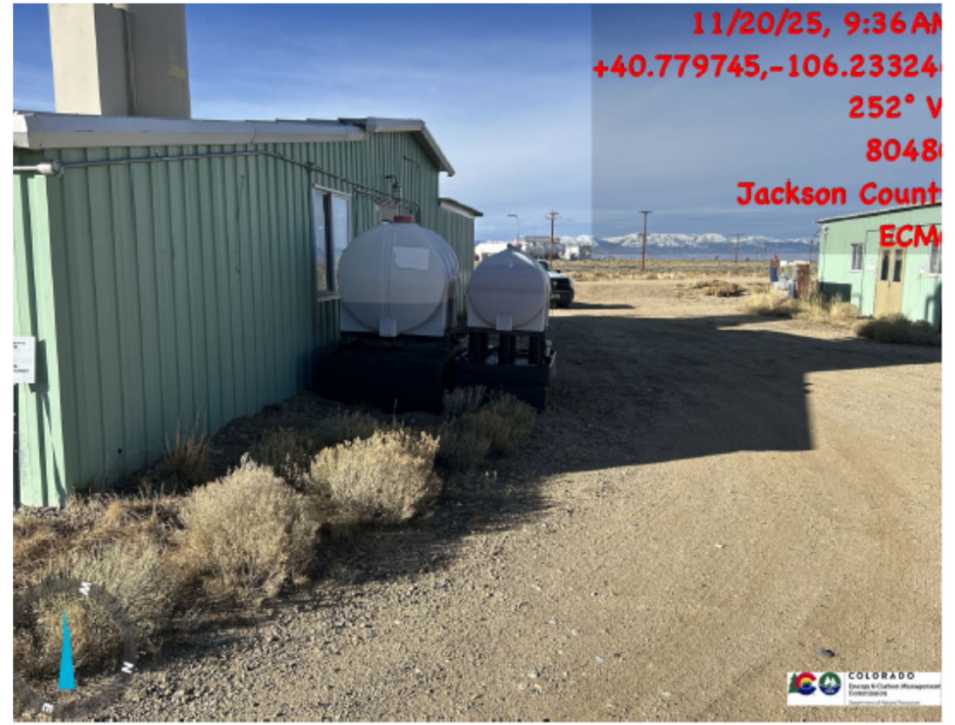
Previous inspection /audit of illegible tank labeling
