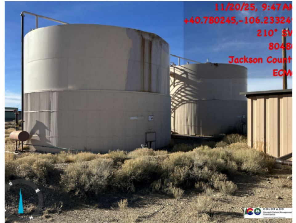
Previous inspection/audit of crude tanks and fiberglass patch
