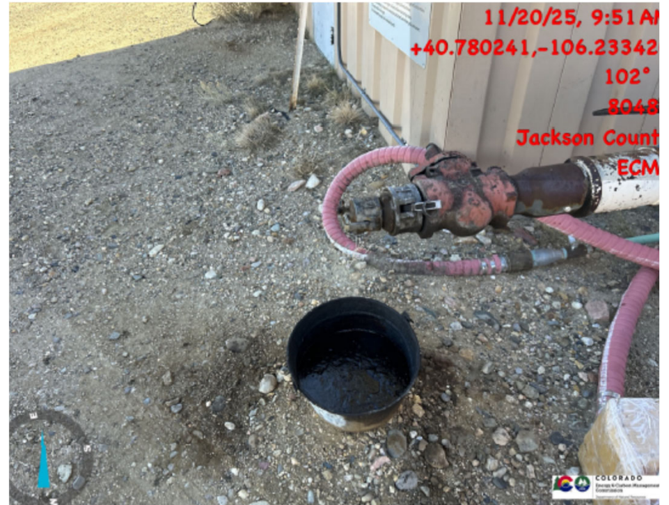
Previous inspection/audit of bucket with crude and staining
