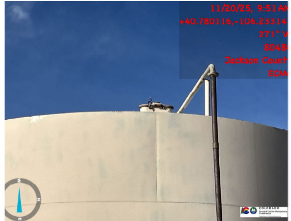
Previous inspection /audit of thief hatch being held shut with a C-clamp, lack of mechanical integrity.
