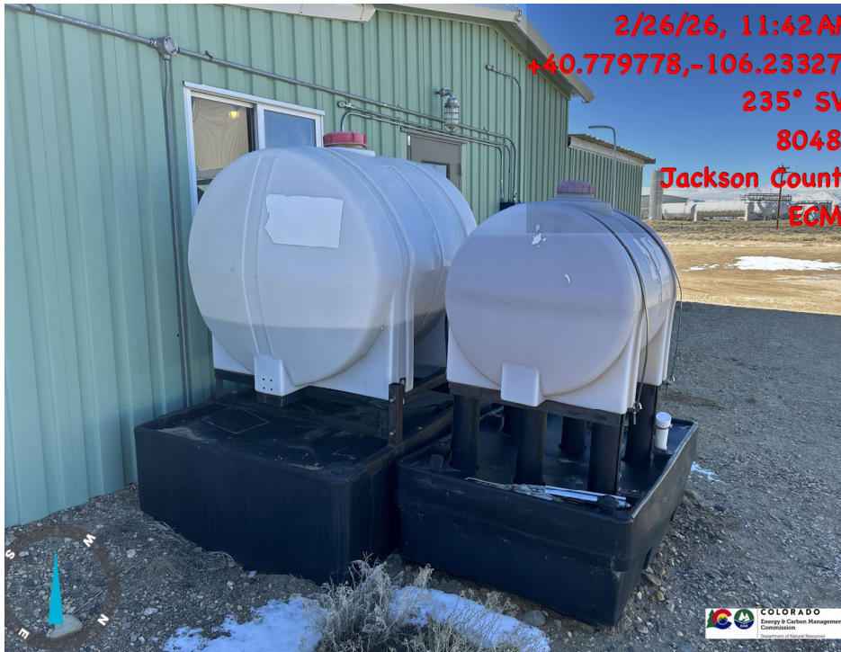
Recent inspection /audit of illegible tank labeling
