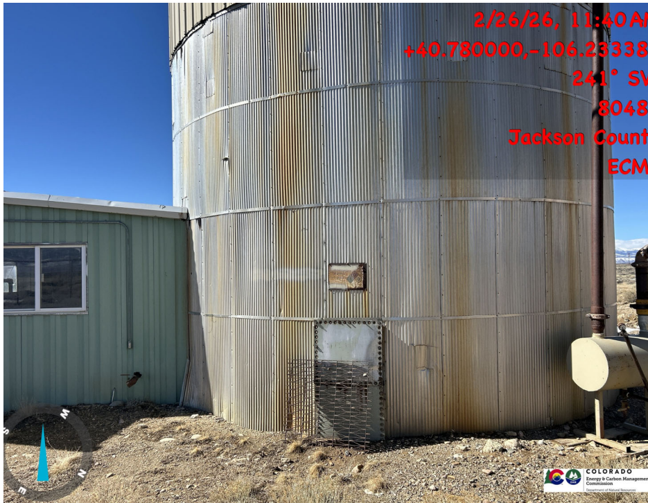
Recent inspection /audit of illegible tank labeling and debris
