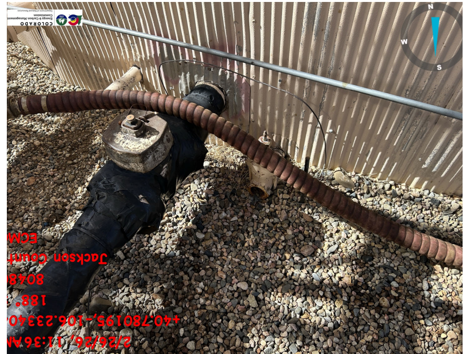
Load line not capped
