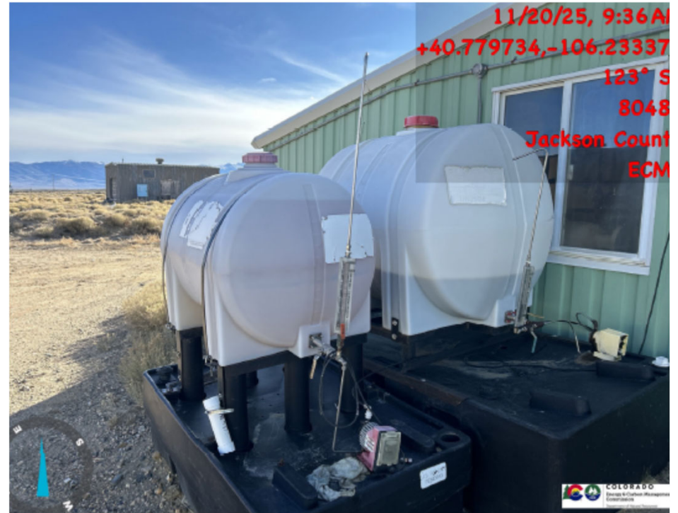
Previous inspection /audit of illegible tank labeling
