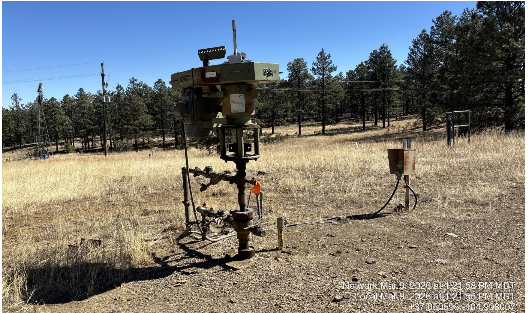
PHOTO 5: 29-15 WELLHEAD AND EQUIPMENT.
