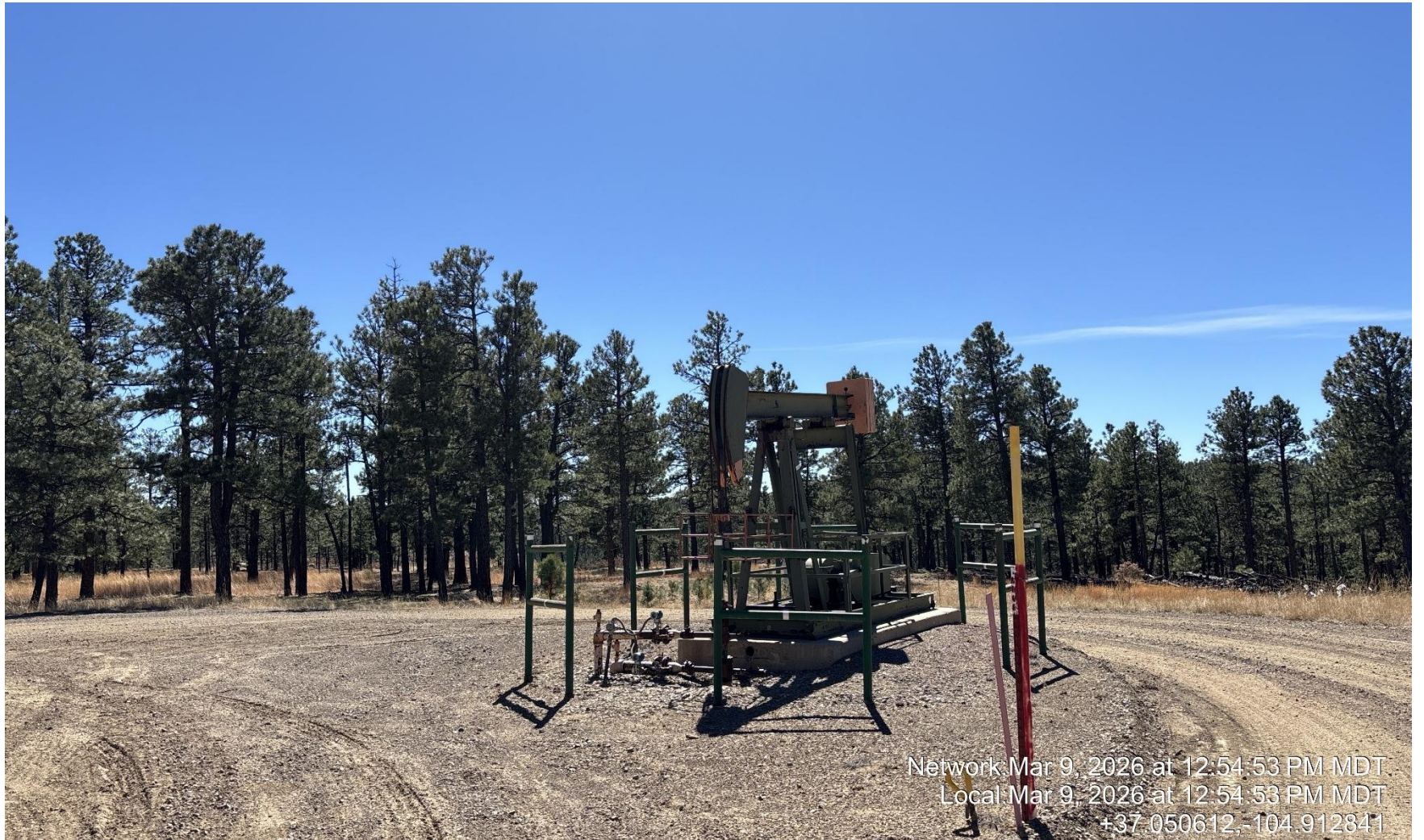
PHOTO 4: WELLHEAD AND EQUIPMENT.
