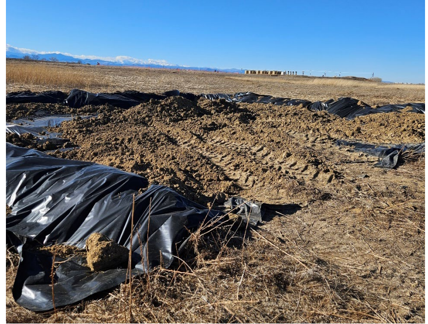
Liner with partial berm adjacent to spill location. Liner has been driven over by equipment.
