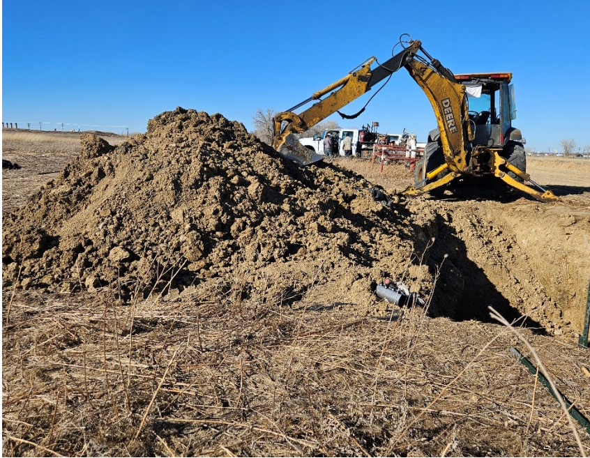
Soil excavated, stockpiled with no liner or stormwater BMPs.
