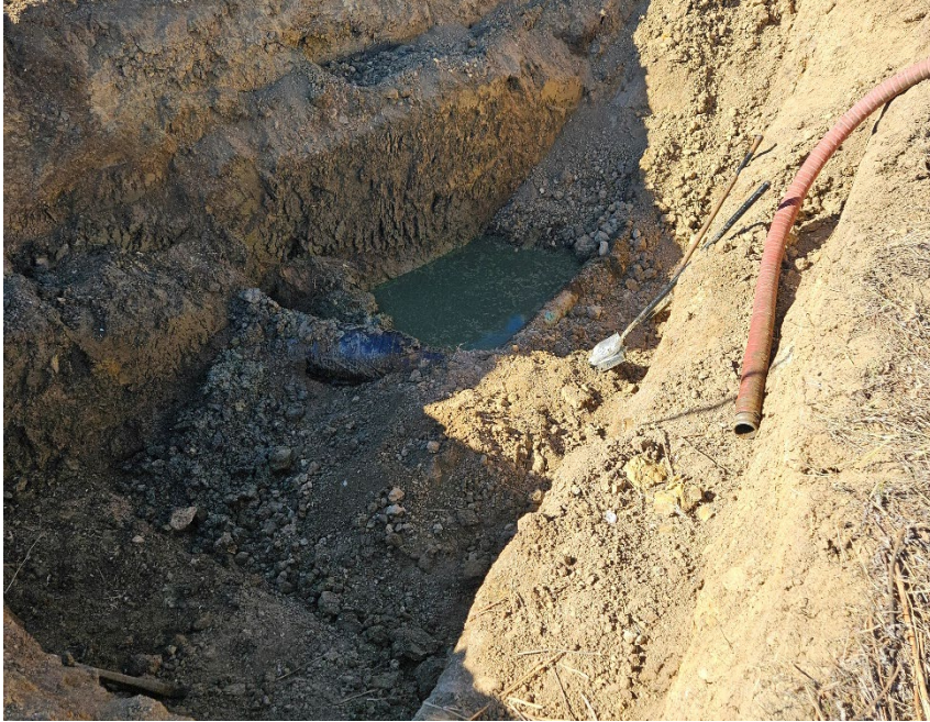
Free product visible at bend in flowline at the base of the excavation.
