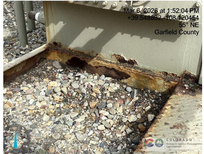
Photo # 7287 External corrosion visible on separator & staining near separator
