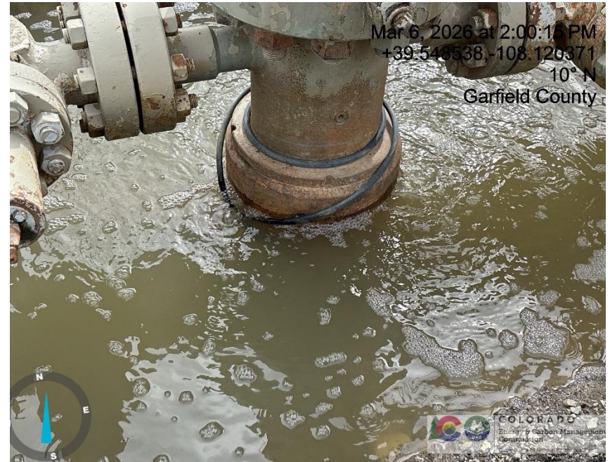
Photo # 7283 Leak/bubbling around CHEVRON 44-5D wellhead
