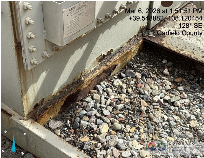
Photo # 7286 External corrosion visible on separator & staining near separator
