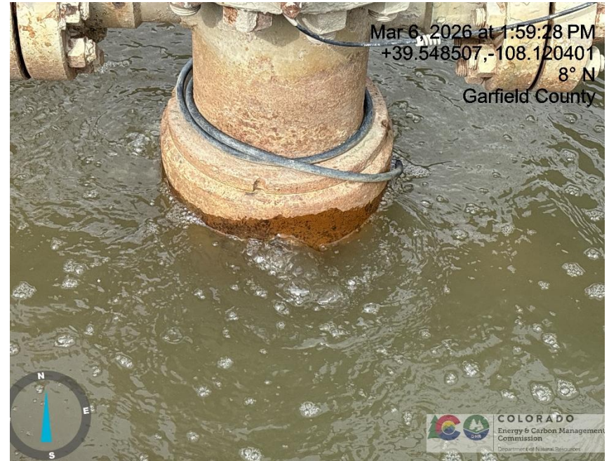
Photo # 7279 Leak/bubbling around CHEVRON 44-5D wellhead
