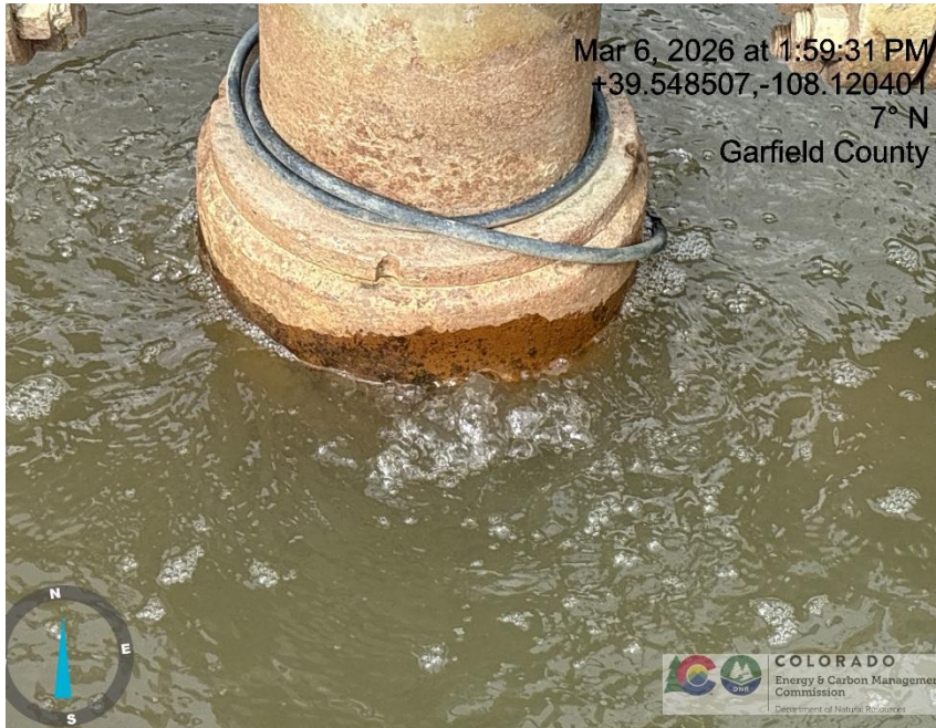
Photo # 7280 Leak/bubbling around CHEVRON 44-5D wellhead
