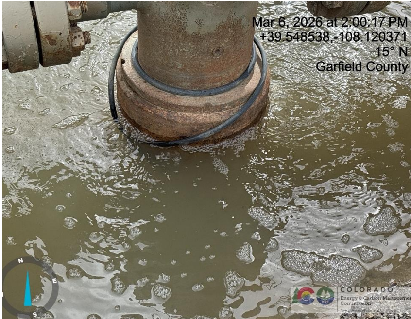
Photo # 7284 Leak/bubbling around CHEVRON 44-5D wellhead
