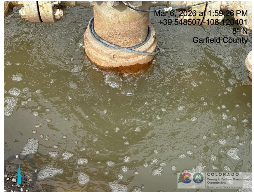
Photo # 7277 Leak/bubbling around CHEVRON 44-5D wellhead
