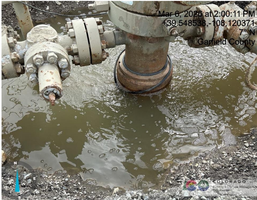
Photo # 7282 Leak/bubbling around CHEVRON 44-5D wellhead
