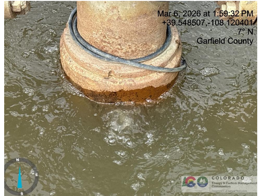
Photo # 7281 Leak/bubbling around CHEVRON 44-5D wellhead
