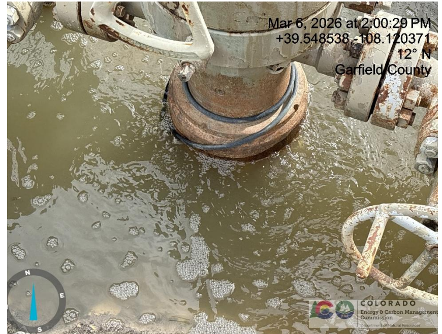
Photo # 7285 Leak/bubbling around CHEVRON 44-5D wellhead
