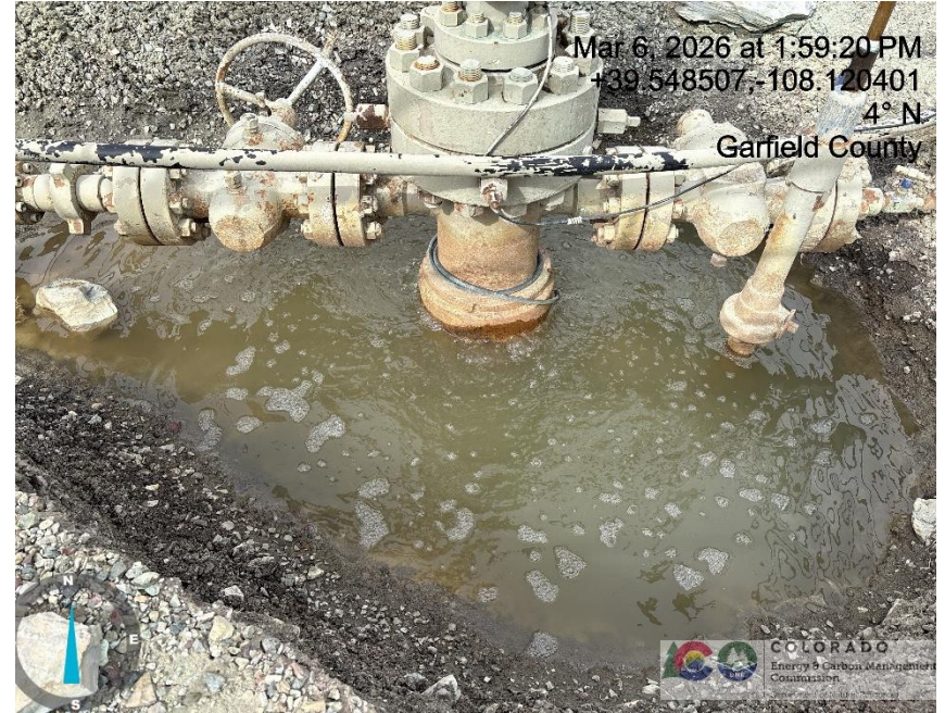
Photo # 7275 Leak/bubbling around CHEVRON 44-5D wellhead
