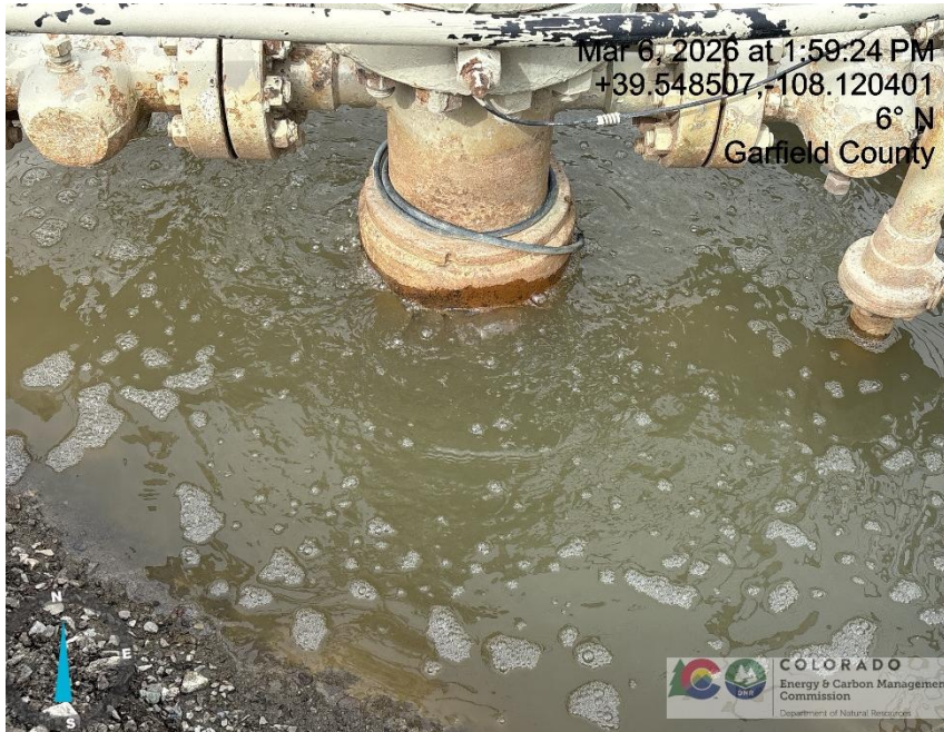
Photo # 7276 Leak/bubbling around CHEVRON 44-5D wellhead
