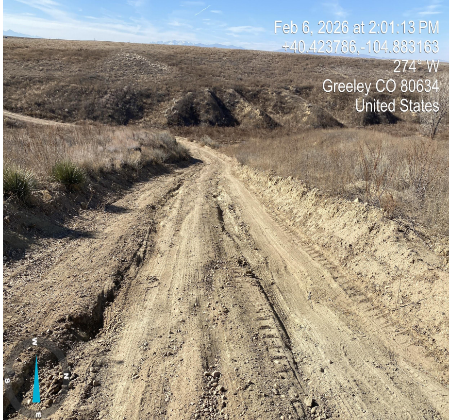
Photo 13. Photo taken from main access road north west past location showing erosion on main road.
