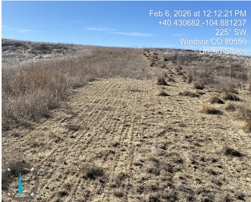
Photo 9. Photo taken of access road facing up slope showing stunted vegetation, areas of bare soil and undesirable annual weeds.
