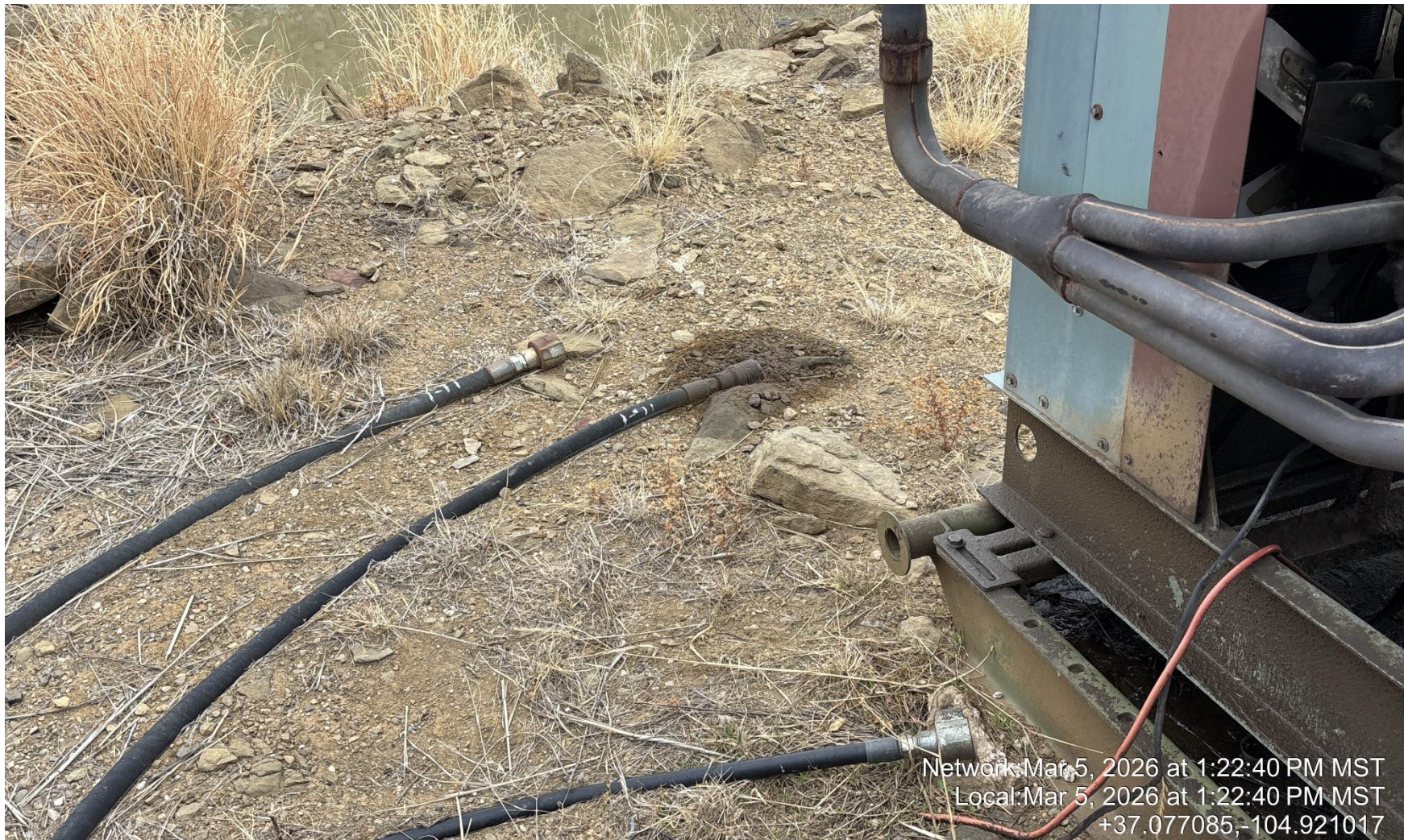
PHOTO 6: AREA OF IMPACTED SOIL FROM PRIME MOVER HYDRALIC HOSE. Conduct maintenance on equipment, cleanup stained material and review self inspection processes. COMPLY WITH RULE 1002,(2).D. CA DATE 3/12/2026.
