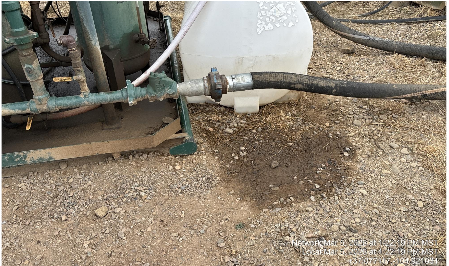
PHOTO 5: AREA OF IMPACTED SOIL NEAR COMPRESSOR. Conduct maintenance on equipment, cleanup stained material and review self inspection processes. COMPLY WITH RULE 1002,(2).D. CA DATE 3/12/2026.
