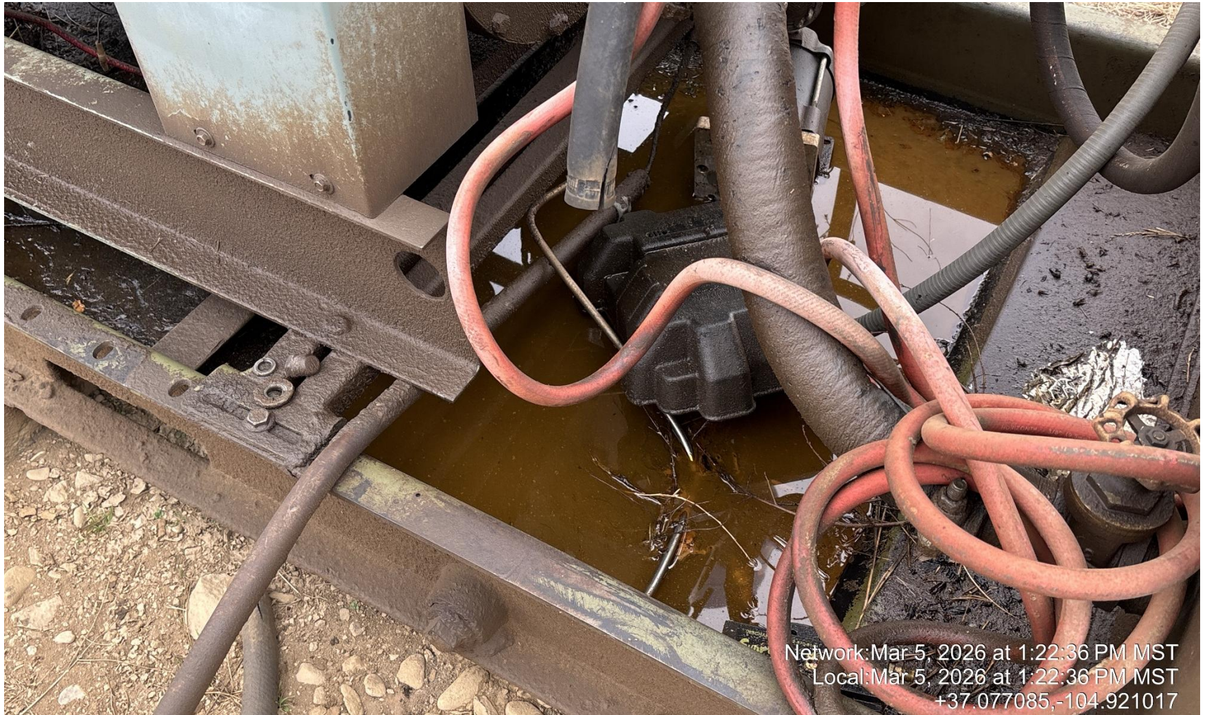
PHOTO 9: OILY WASTE IN PRIME MOVER ENGIN SKID WITHOUT WILDLIFE PROTECTION SCREENS OR NETTING. DRAIN OILY WASTE REPAIR ALL LEAKS AND REMOVE IMPACTED SOIL PER RULE 1002..(2).D & 1002.f.(2)B, Comply with general provisions of the oil and gas act for wildlife protection AND SB-181. CA DATE 24 HOURS TO DRAIN OILY WASTE OR INSTALL WILDLIFE PROTECTION 3/12/2026 FOR ANY IMPACTED SOILS.
