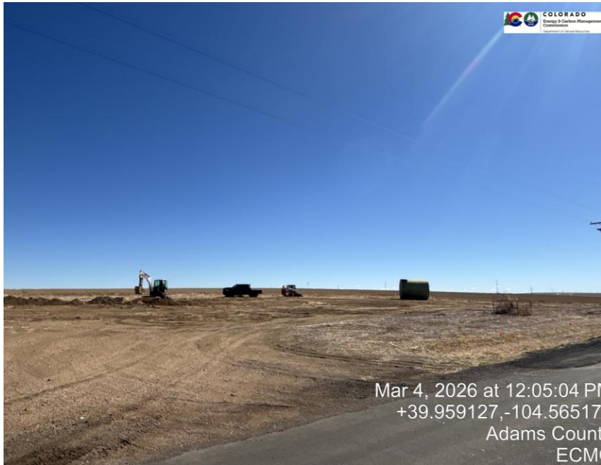
Pic 3 tank battery has been removed, one tank remains, ready to be removed.
