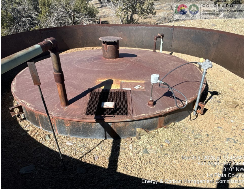
NO TANK OR BERM PAINT
