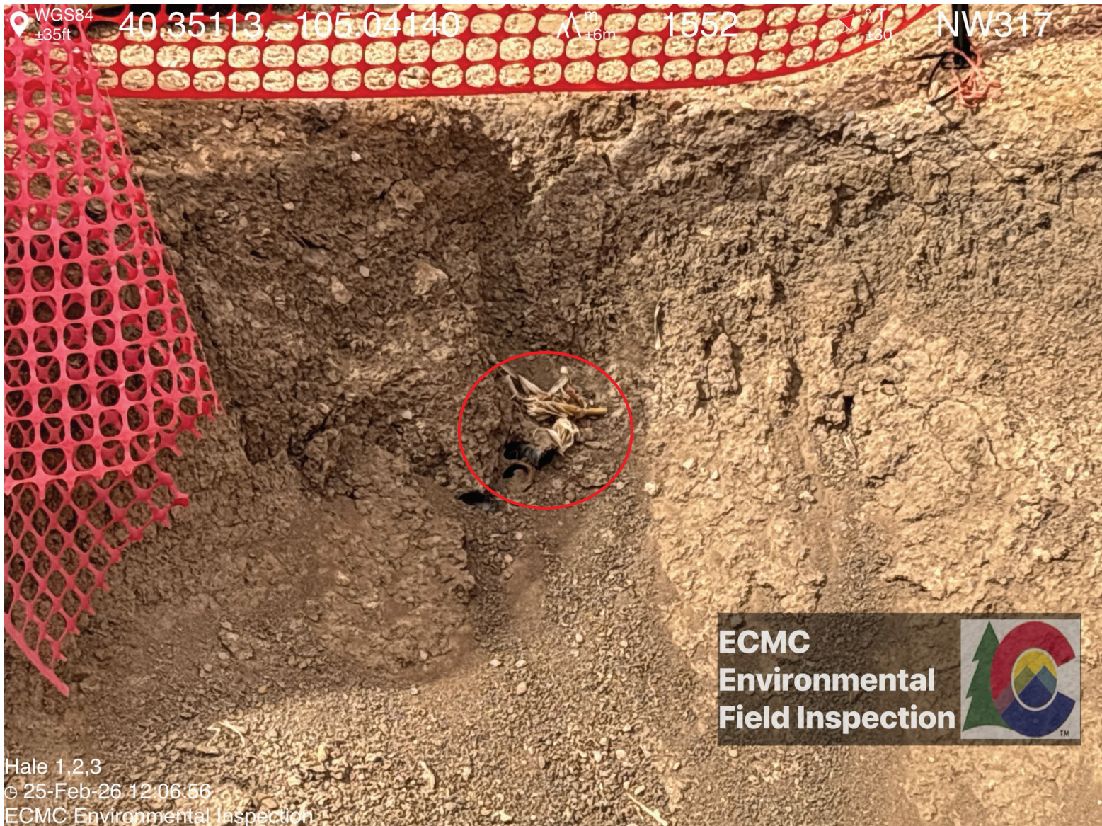
Uncapped flowlines visible in sidewall of the northwest corner of the open excavation
