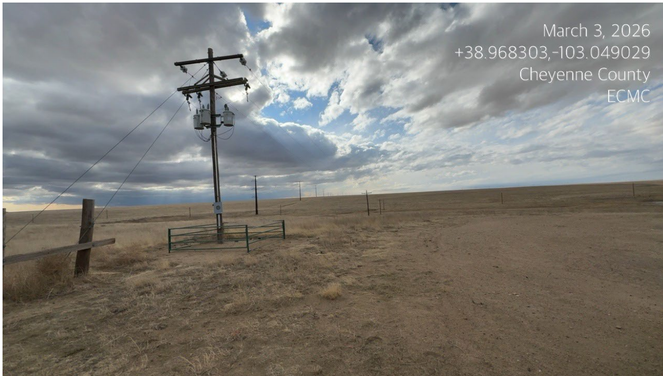
Photo 5. The powerline servicing the former wellsite needs to be removed
