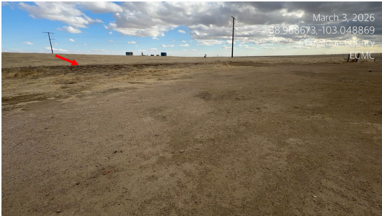
Photo 4. Facing southeast at the location. There is a cut slope at the red arrow where soil needs to be recontoured back to the terrain.
