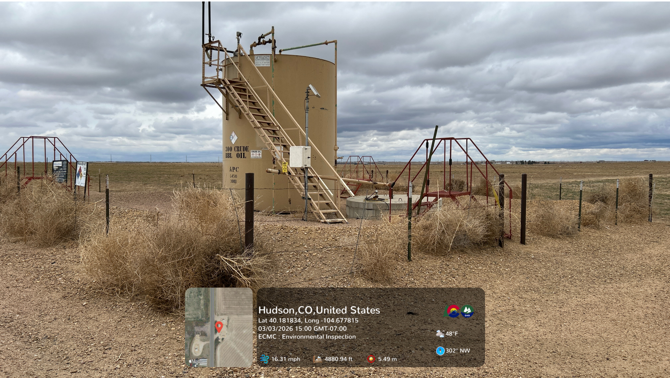
Looking at production tank and produced water vessel containment. Debris is visible around the metal wire fence.
