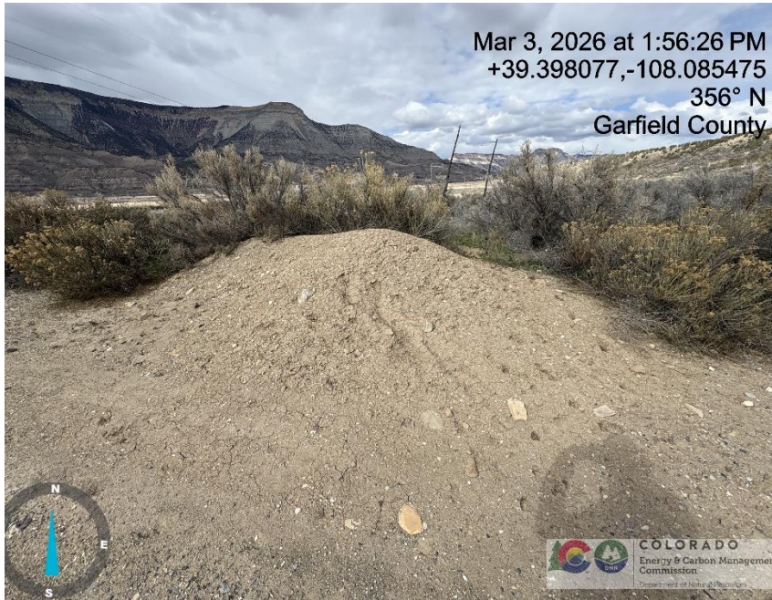
Photo # 5190 Soil stockpile lacks BMP's
