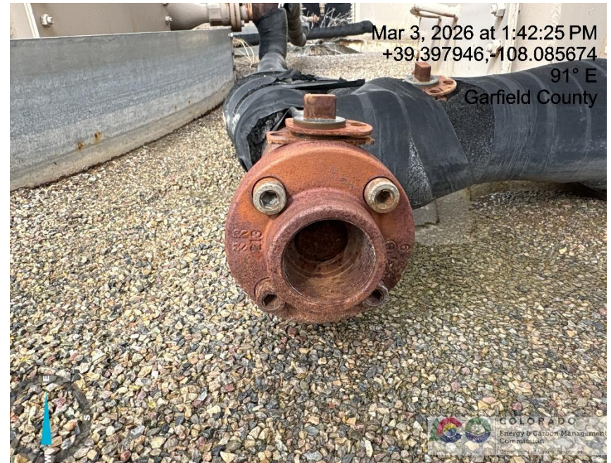
Photo # 5175 Open ended load line
