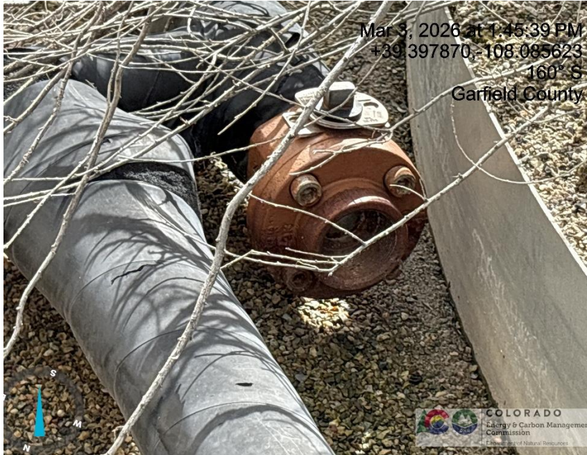
Photo # 5178 Open ended load line
