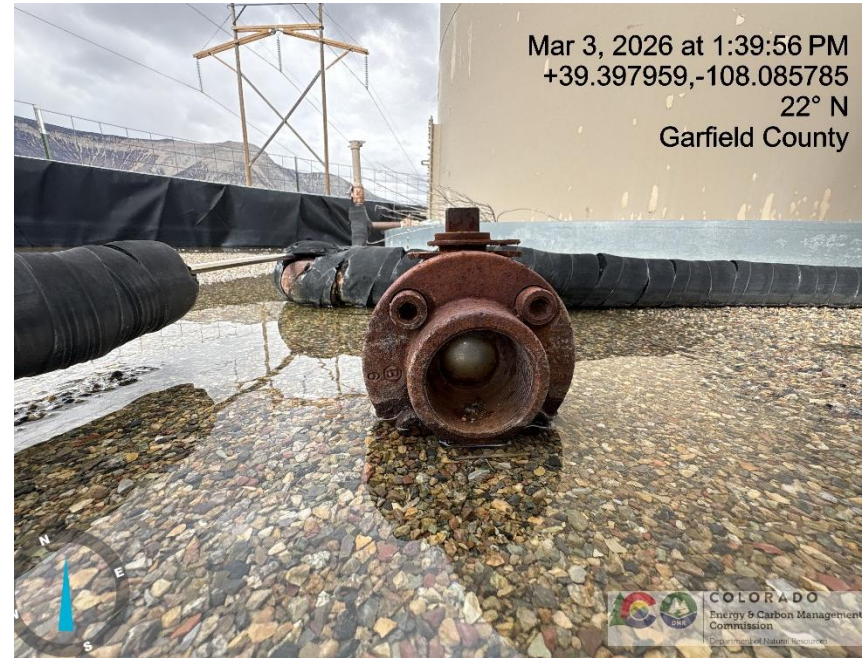
Photo # 5173 Open ended load line
