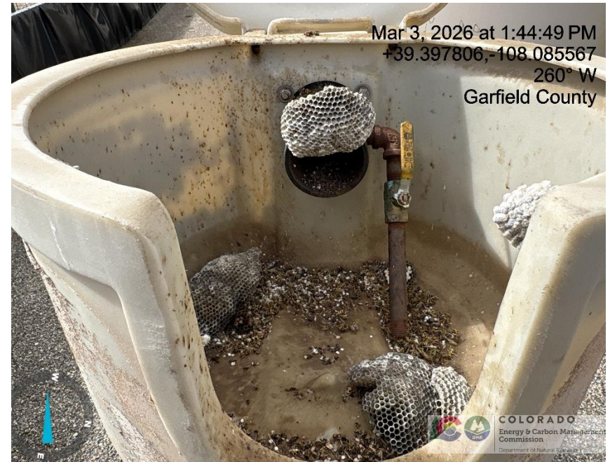
Photo # 5177 Open ended load line
