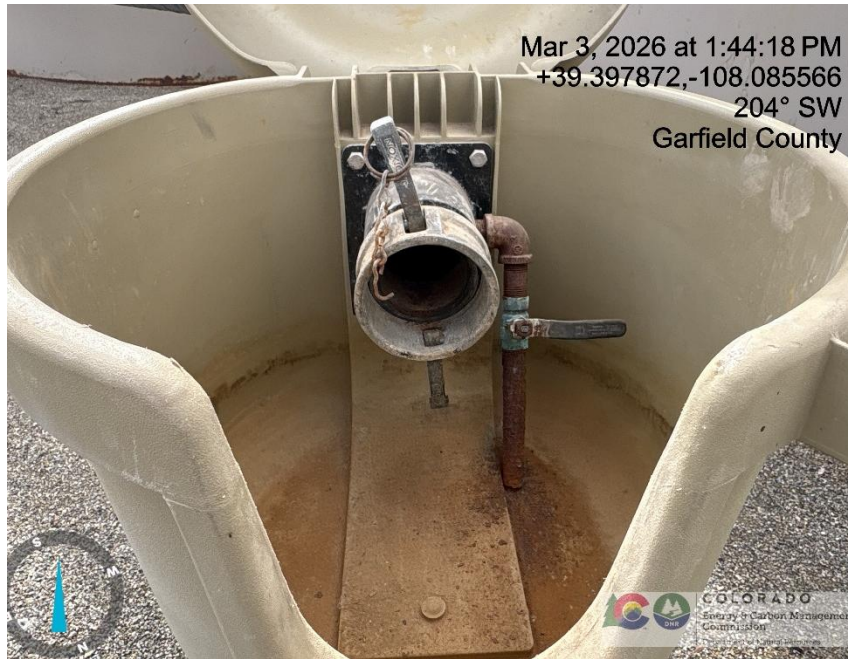
Photo # 5176 Open ended load line
