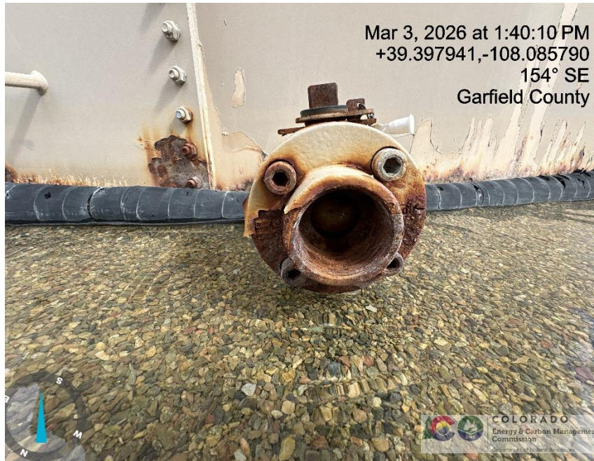
Photo # 5174 Open ended load line
