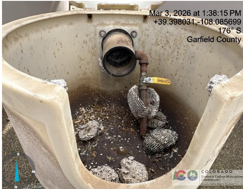
Photo # 5172 Open ended load line
