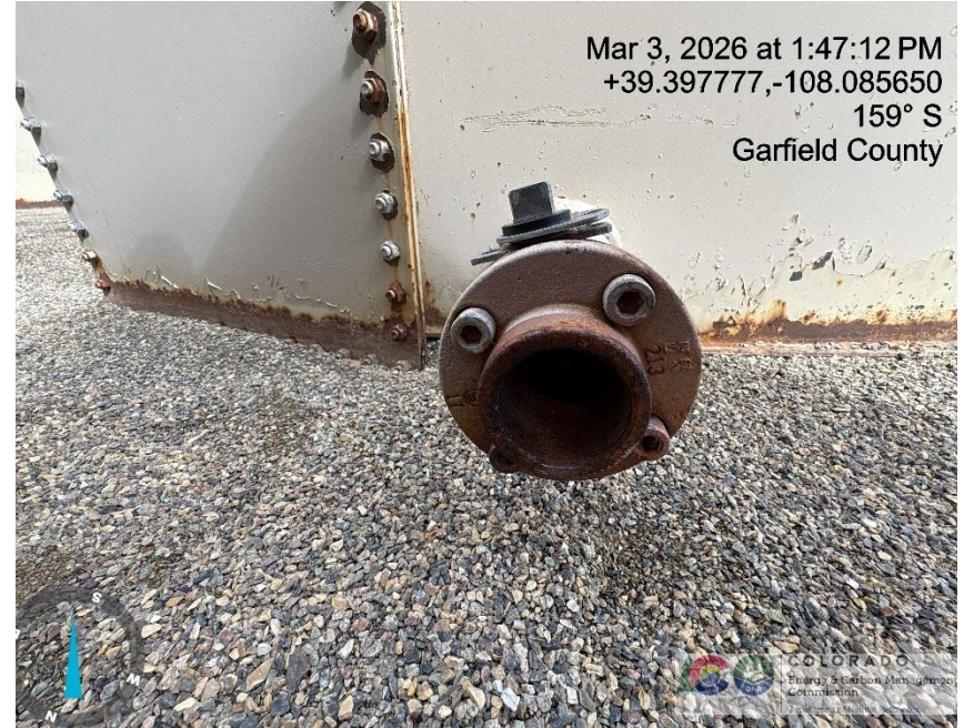
Photo # 5179 Open ended load line
