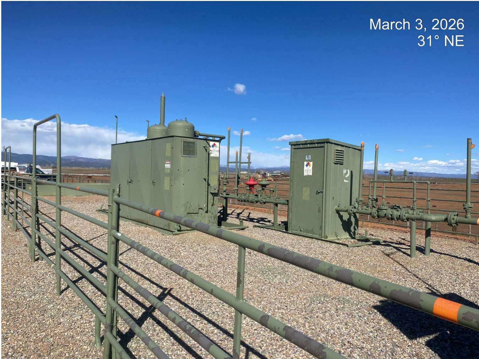
Photo 2. View of equipment and labels on the eastern edge of the pad.
