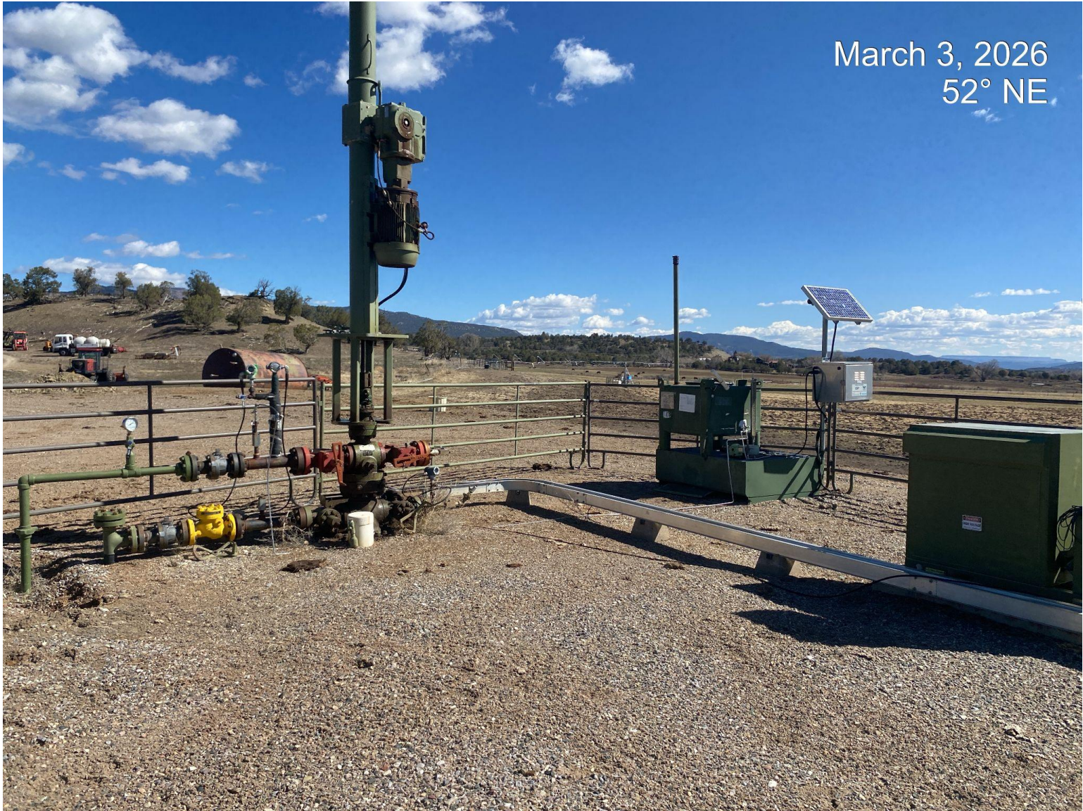
Photo 2. View of wellhead assembly equipment.
