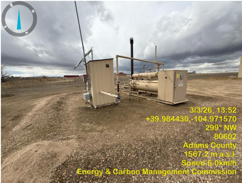
Photo 9 Separator, Gas Meter Run.
