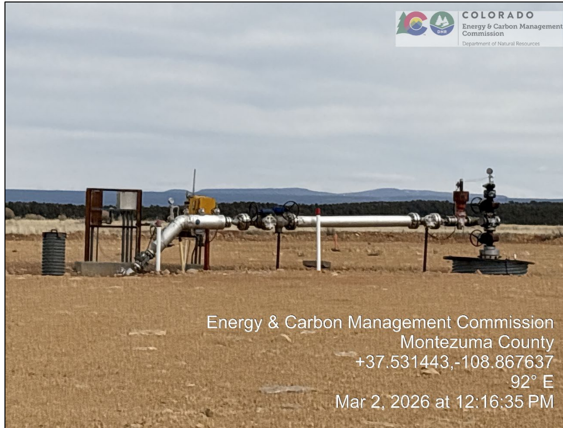
3. Wellhead, cellar, insulated flow line, telemetry and electrical controls, CP test points, and corrugated pipe used for hose storage. View looking due east.
