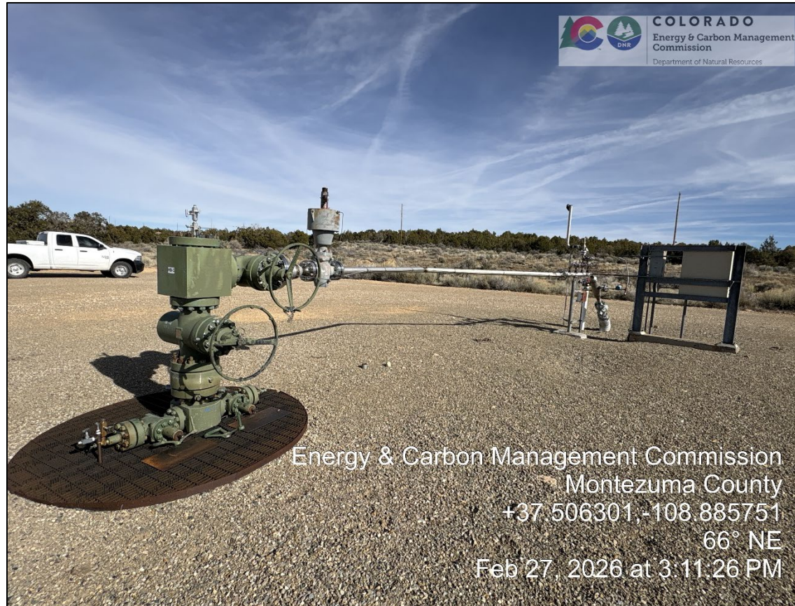
2. Wellhead, cellar, flow line and electrical controls.
