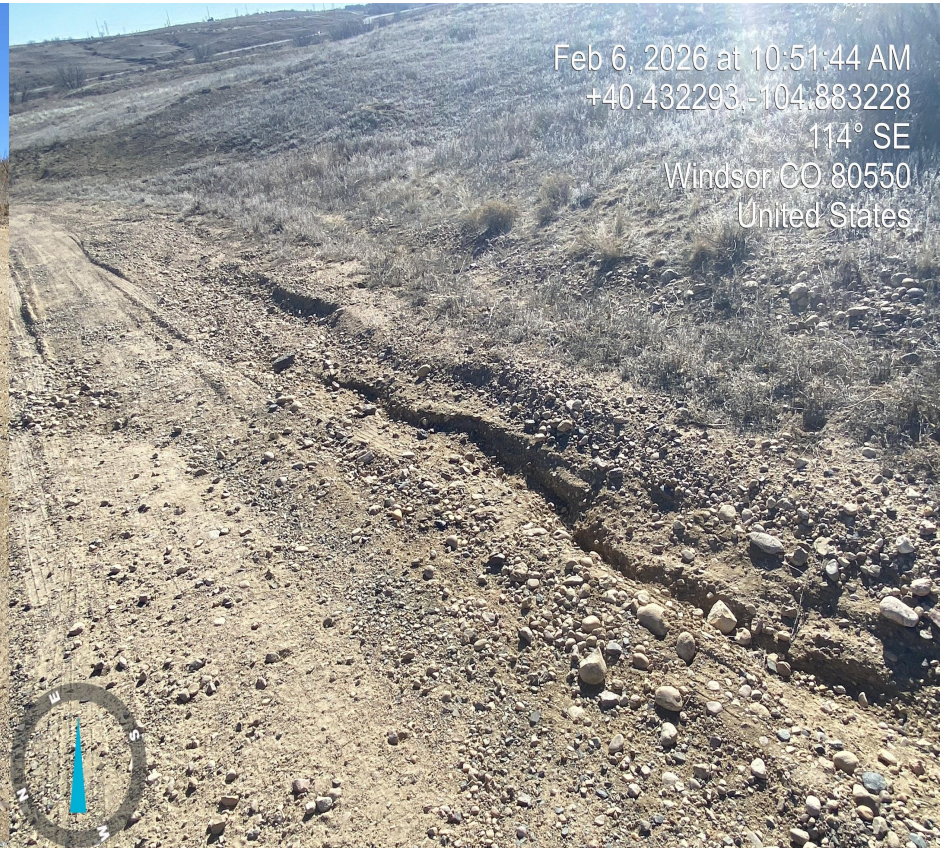
Photo 14. Photo shows erosion on main access road.
