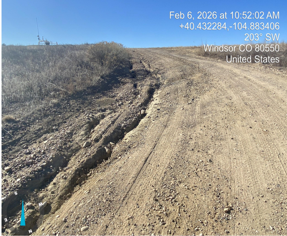
Photo 15. Photo shows erosion on main access road.
