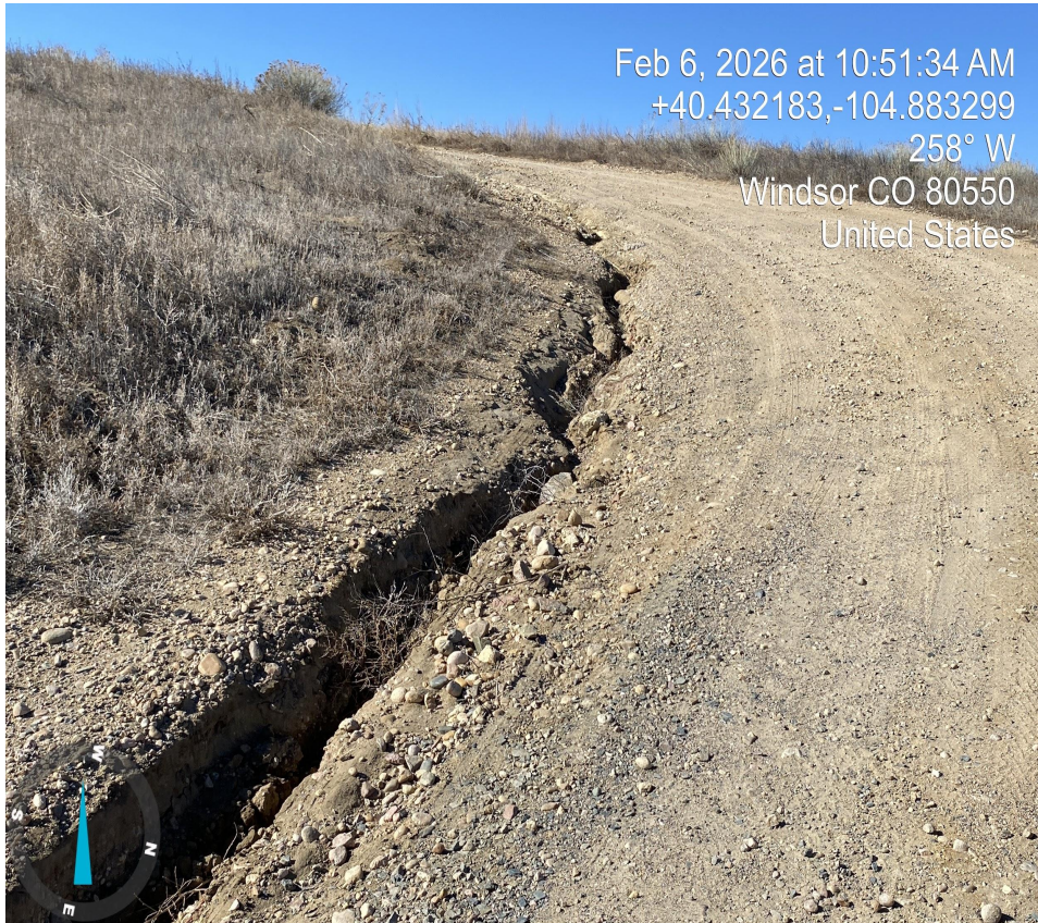
Photo 13. Photo shows erosion on main access road.
