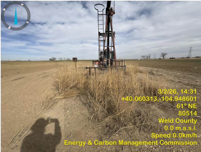
Photo 9 Wellhead overrun with dead vegetation.
