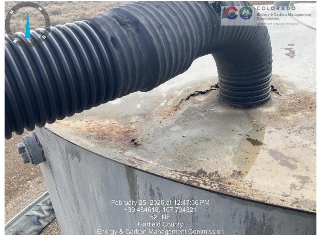
Rusted out tank top
