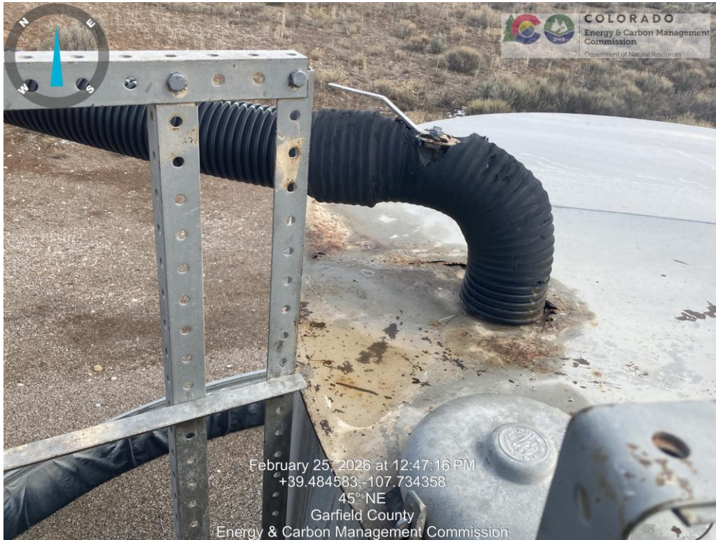
Rusted out tank top
