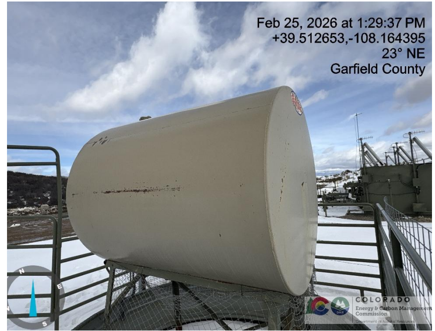
Photo # 4033 Methanol tank lacks operator name & 911
