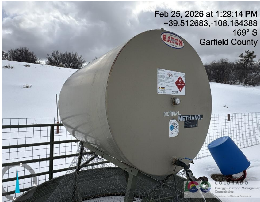
Photo # 4032 Methanol tank lacks operator name & 911
