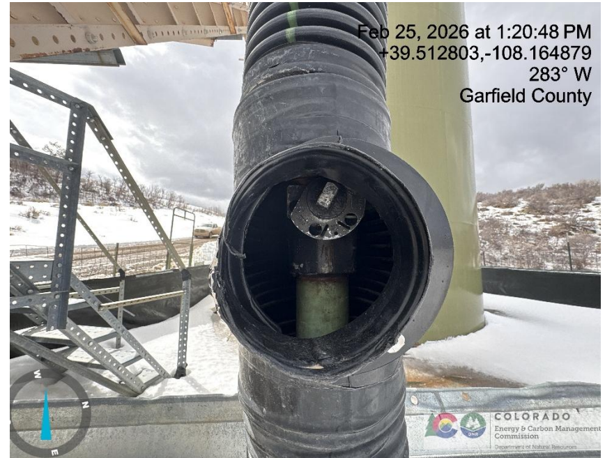
Photo # 4035 Flowline heating insulation open ended /wildlife hazard/available for entry by wildlife
