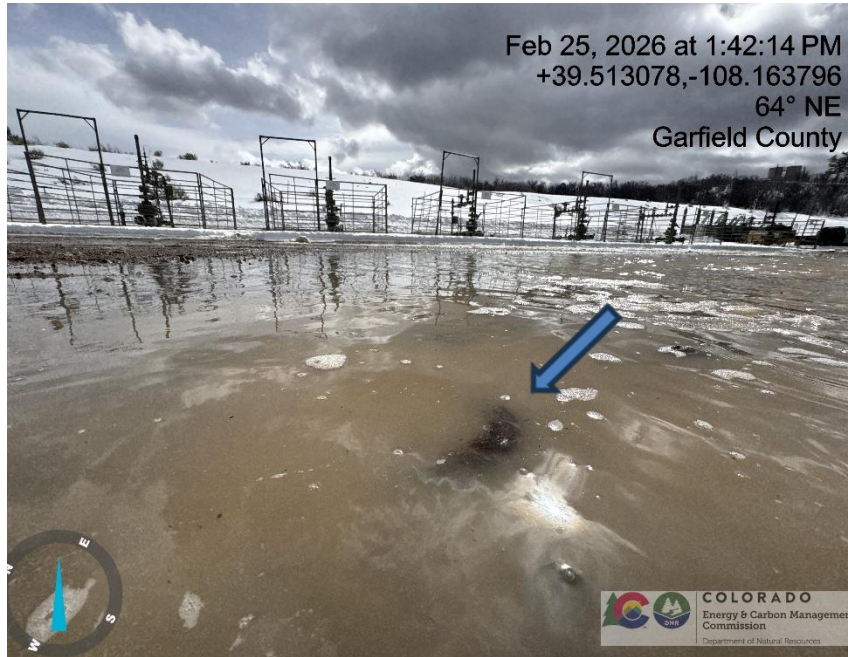
Photo # 4038 Same unmarked deadman
