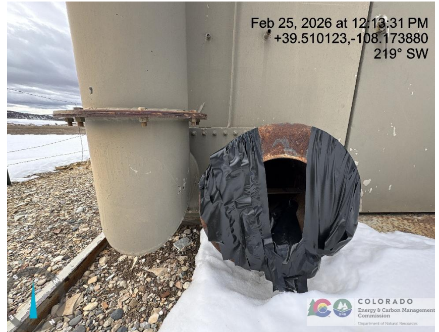
Photo # 3756 Fire tube open ended/wildlife hazard /available for entry by wildlife
