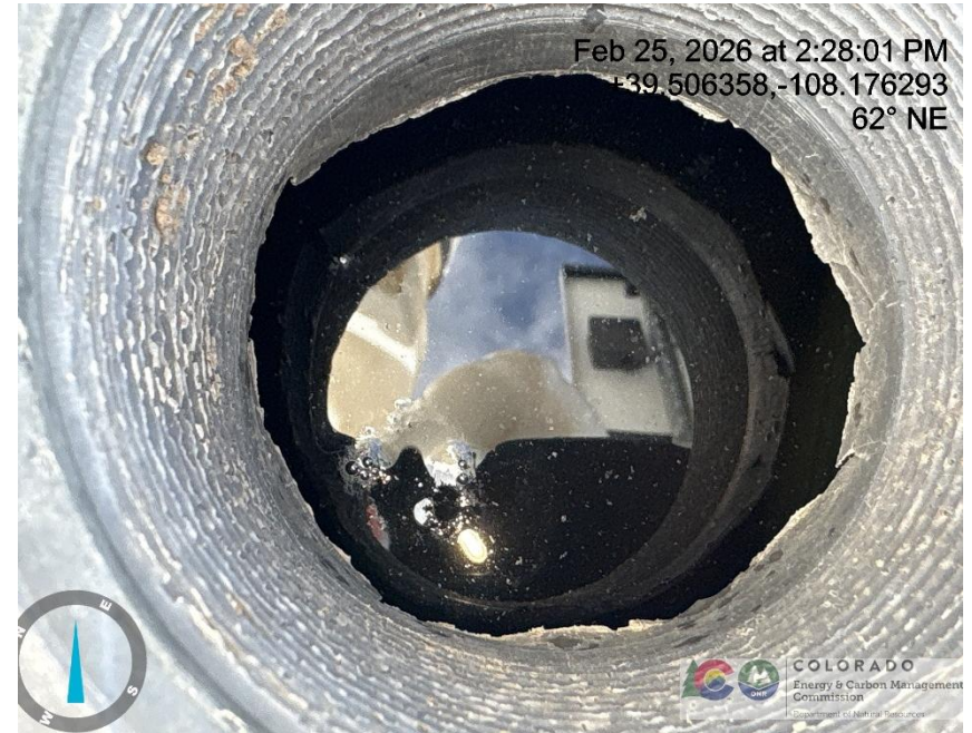
Photo # 4177 Failure to maintain chemical BMP – Chemical tank containment approximately 3/4 to 7/8 full of fluid/BMP insufficient to contain possible spill
