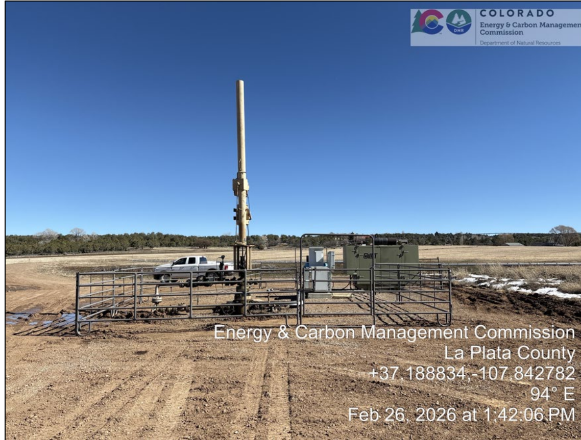
03. Wellhead and electric drive progressive cavity pump along with electrical controls.
