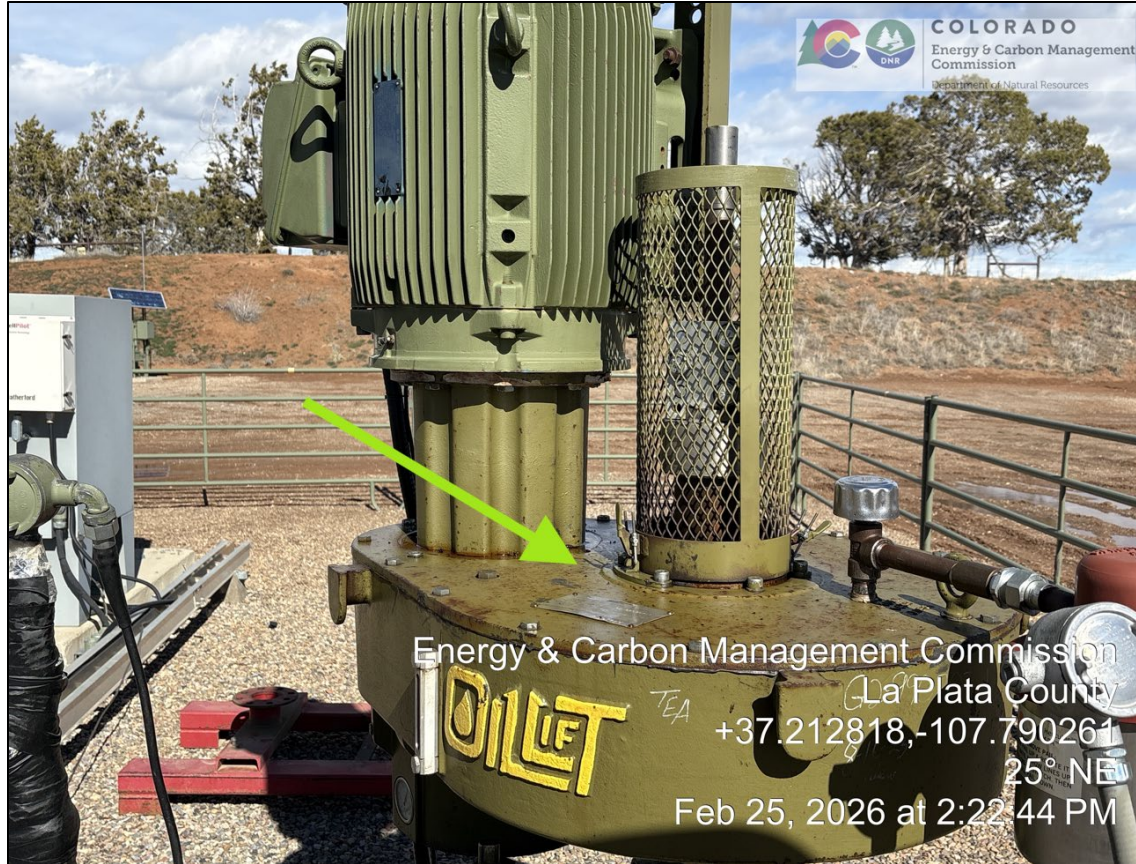
14. Hester 2 electric-drive progressive cavity pump. The yellow arrow points at the oil accumulated on rod oiler which is dripping down onto gravel.
