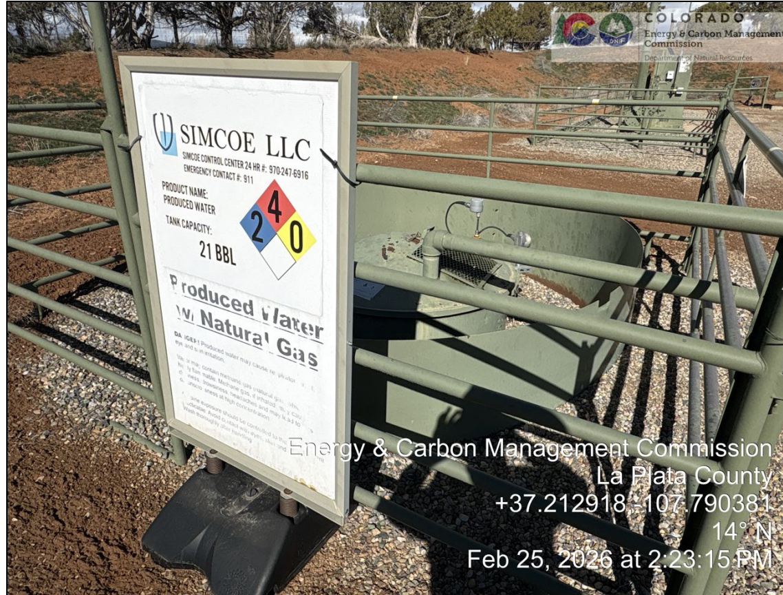
15. Hester 2 produced water with natural gas 21 bbl tank.
