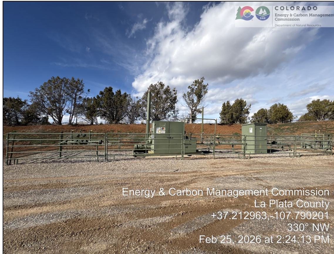
17. Overview of Hester 2 horizontal heated separator, meter run, and 3' flow lines.
