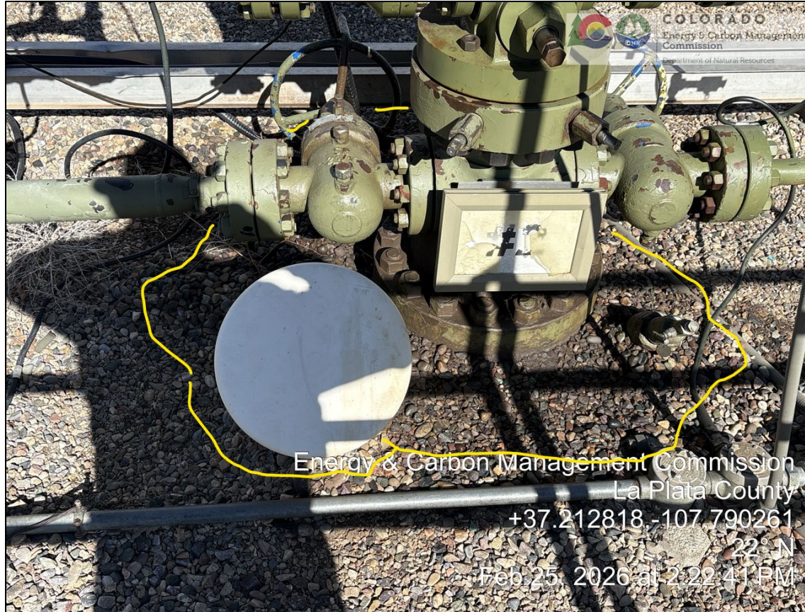
13. Hester 2 wellhead and bradenhead access. Note stained gravel inside of yellow outline.
