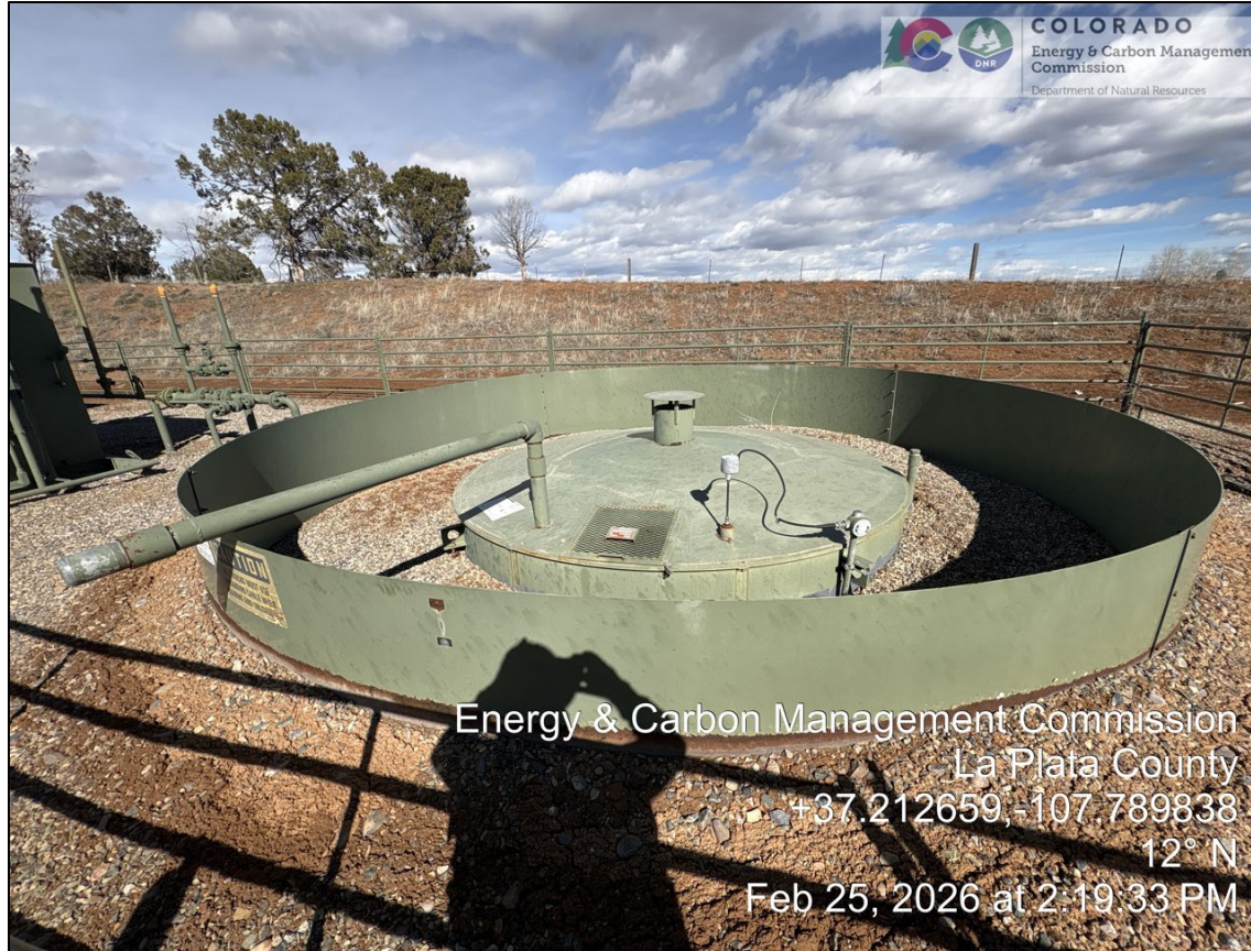
05. Hester 4 95 BBL produced water tank and secondary containment.
