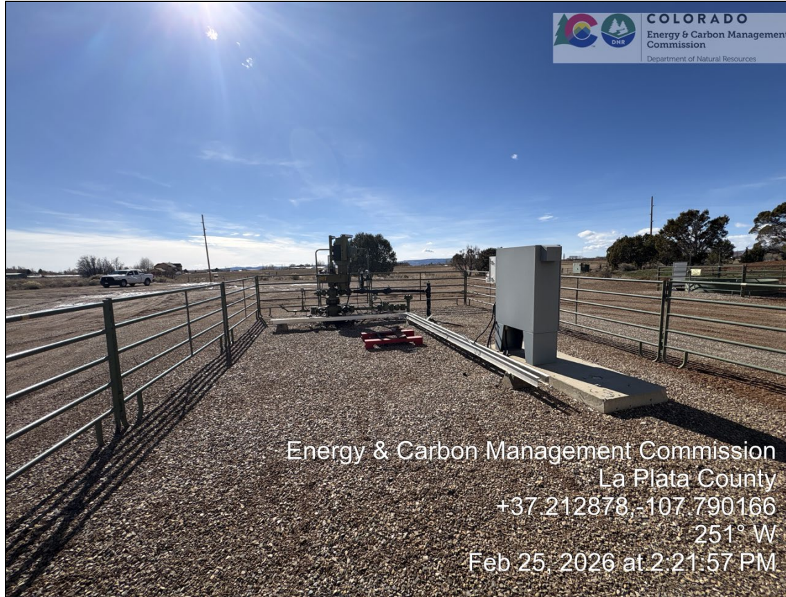
11. Hester 2 wellhead with electric progressive cavity pump.
