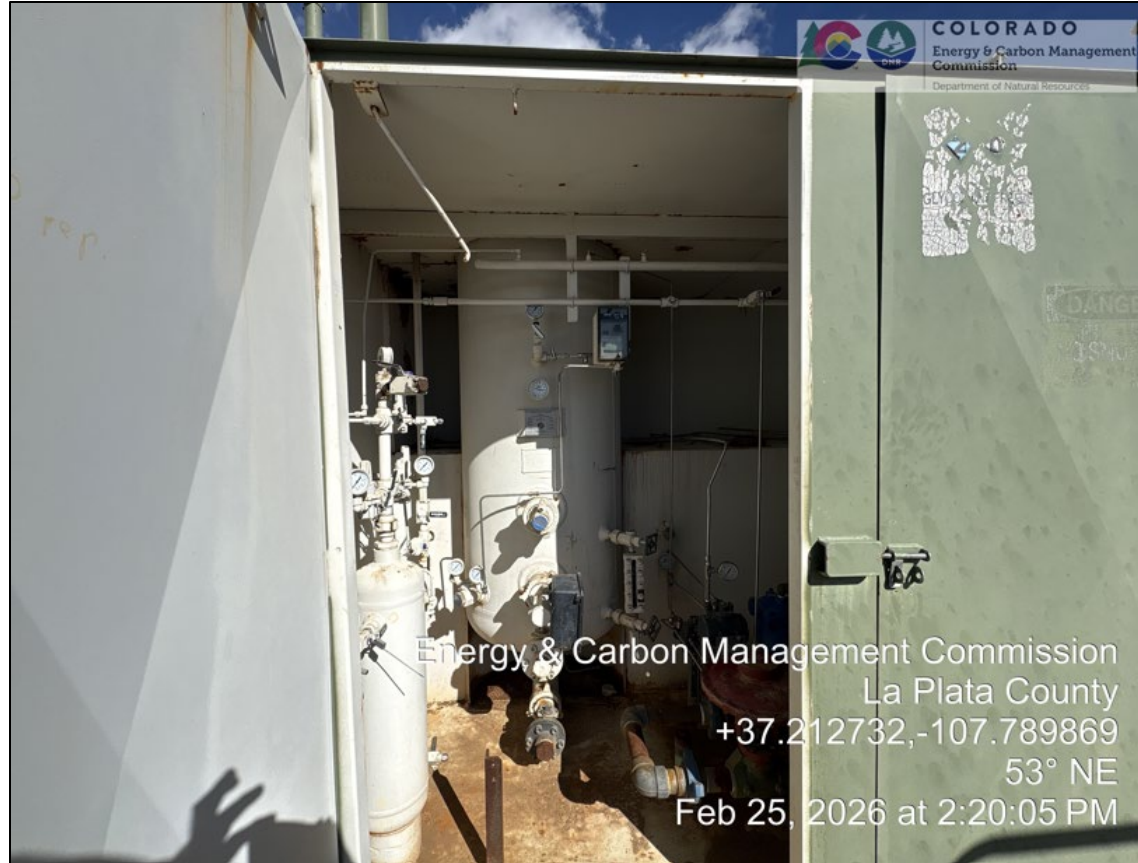
06. Inside Hester 4 vertical heated separator structure.
