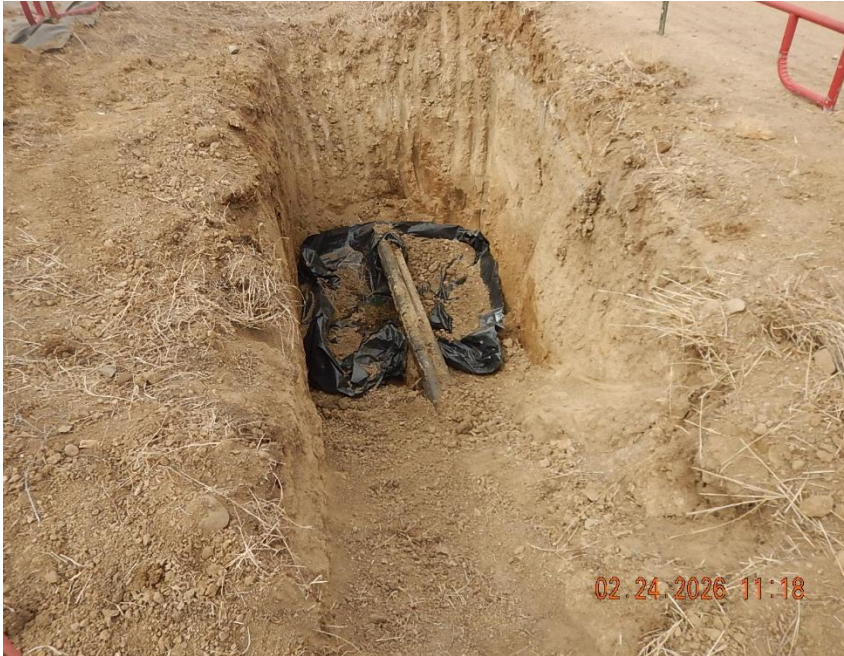
(1) 4" CS off location flowline (Facility 8 consolidation) and (1) 2" CS gas line (OOS) exposed in excavation at point of release (40.049530, -104.866933); poly liner under pipes.
