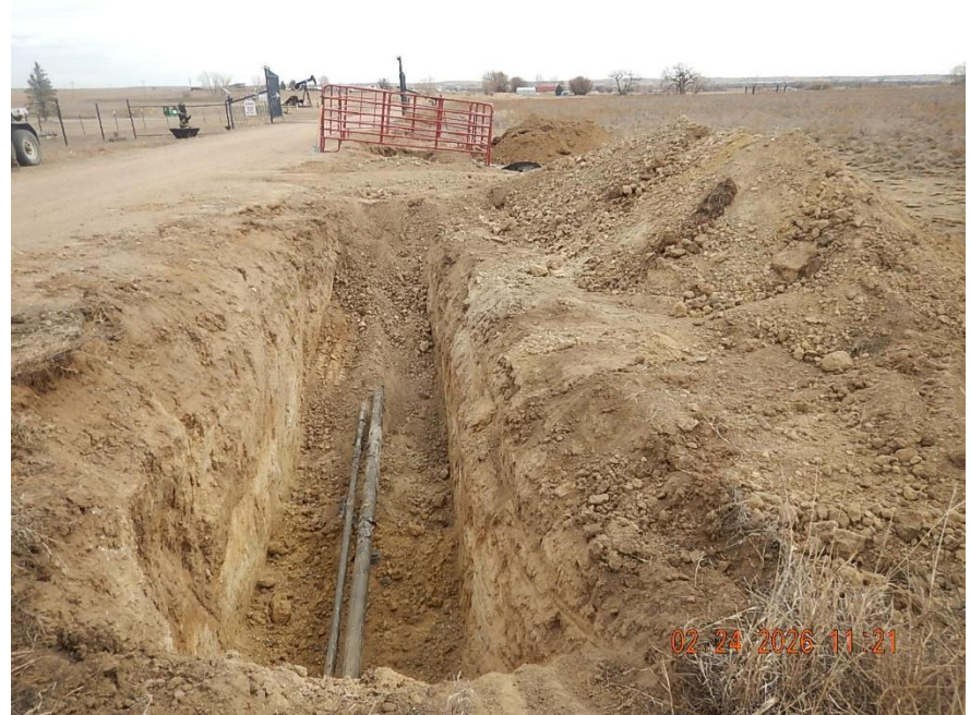
West bell hole excavation @ 40.049530, -104.867144 and Facility 8 off location flowline(s) exposed. View looking east toward fenced spill/ release excavation.
