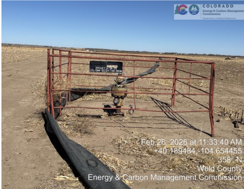
Photo 1 well head and equipment
