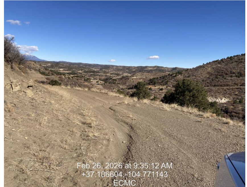
Photo 6: erosion along access road
