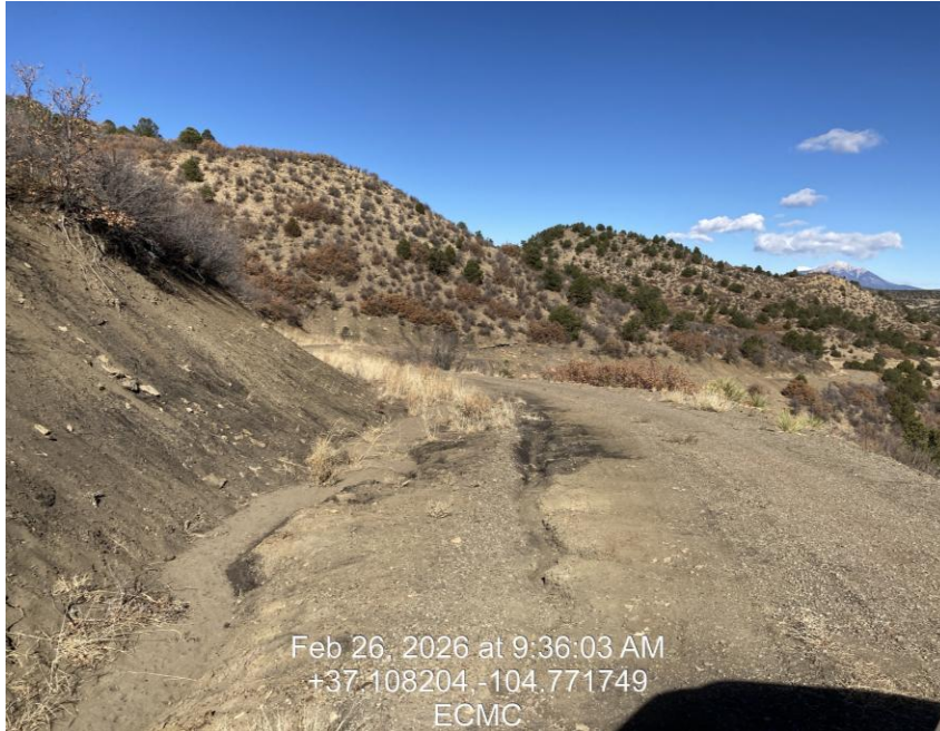
Photo 5: erosion along access road
