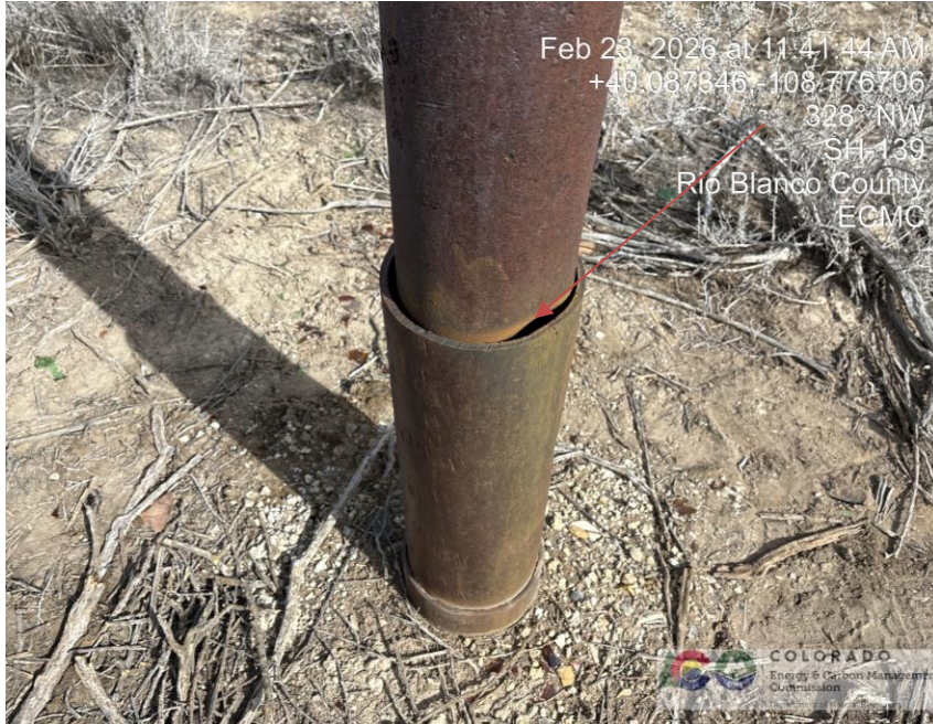
Photo # 2269 Plugged and abandoned well actively venting gas during inspection.
