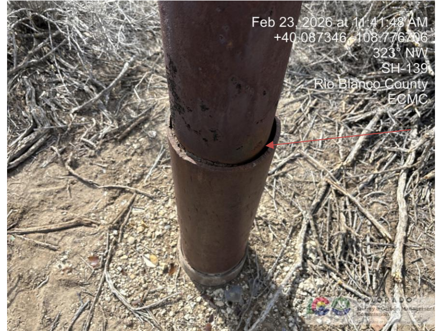
Photo # 2270 Plugged and abandoned well actively venting gas during inspection.
