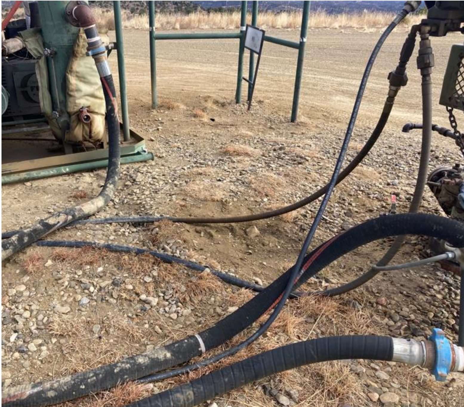
PHOTO 1: THE HYDRAULIC HOSES HAVE BEEN REPAIRED AND ALL OPERATING EQUIPMENT HAS RECEIVED MECHANICAL MAINTENANCE. THE STAINED SOIL UNDER THE WELL HEAD HAS BEEN REMOVED AND REPLACED WITH FRESH PAD MATERIAL.
