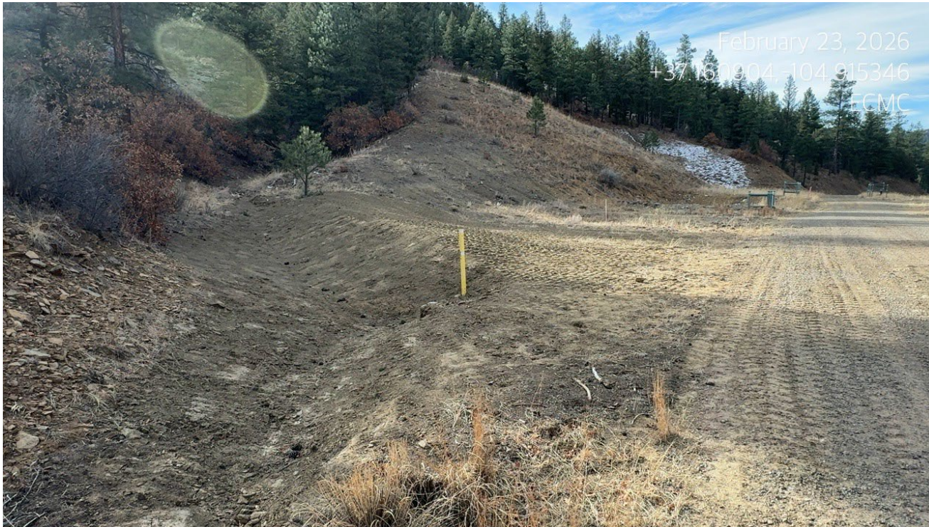
Photo 4. Facing southeast at north side of the location. This area of the culvert has been regraded and reseeded.
