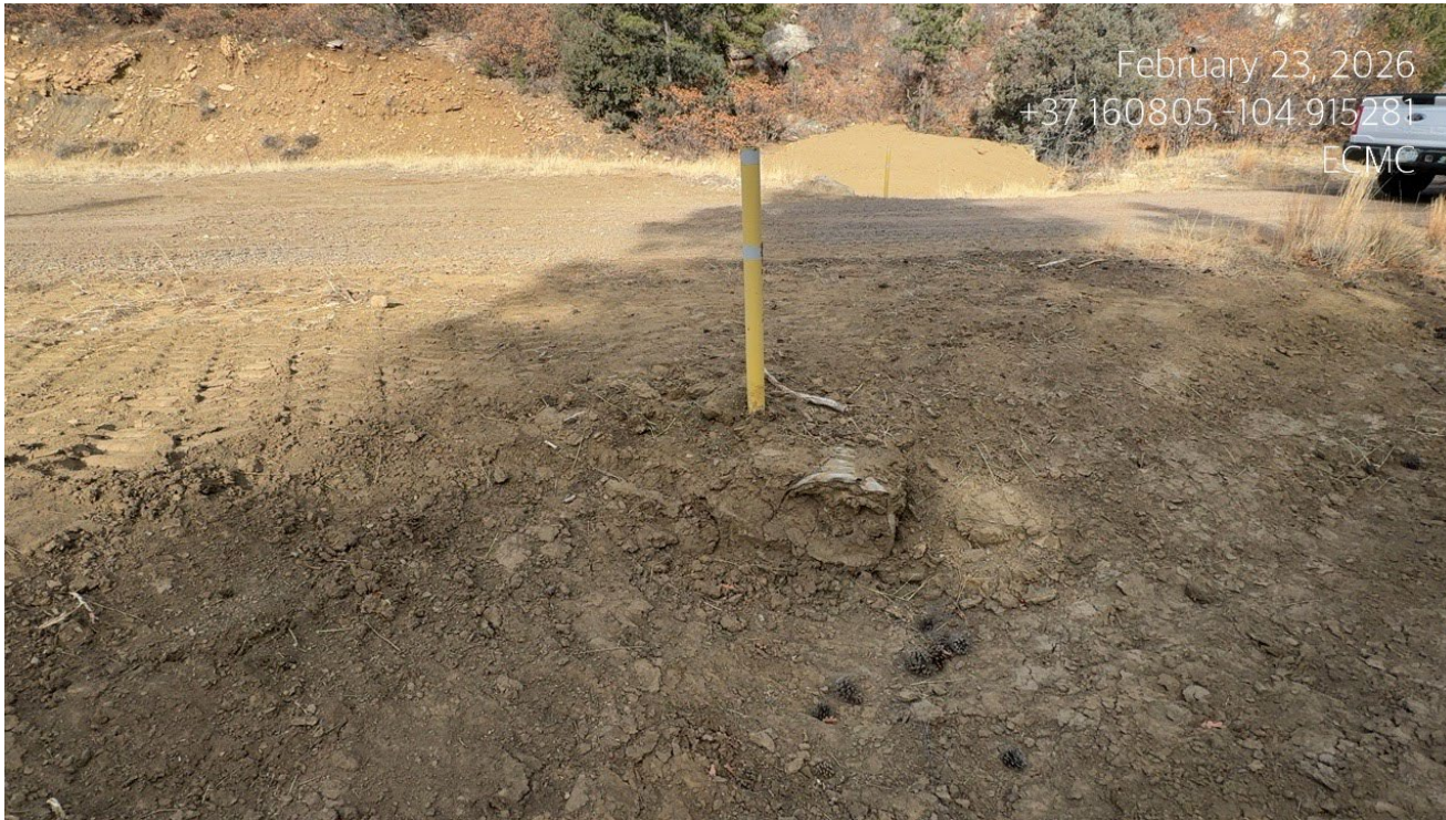
Photo 5. This culvert is filled in with sediment and needs to be cleaned out or replaced..
