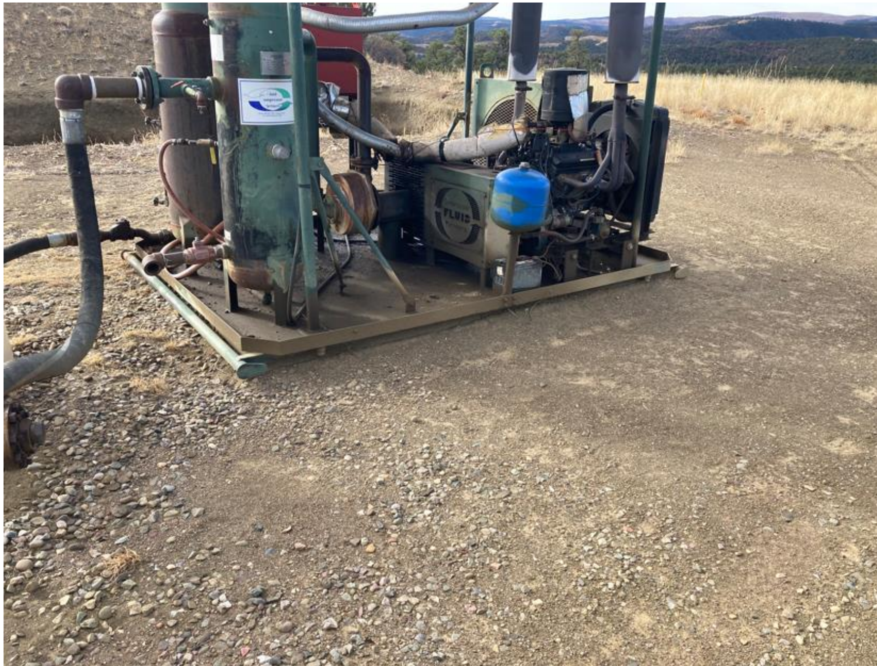
PHOTO 1: THE LEAK HAS BEEN STOPPED ON THE WELL HEAD AND PACKING HAS BEEN TIGHTENED. THE IMPACTED SOIL HAS BEEN REMOVED FROM LOCATION AND REPLACED WITH FRESH PAD MATERIAL. THE SKID HAS BEEN CLEANED AND ALL OPERATING EQUIPMENT HAS RECEIVED MECHANICAL MAINTENANCE.
