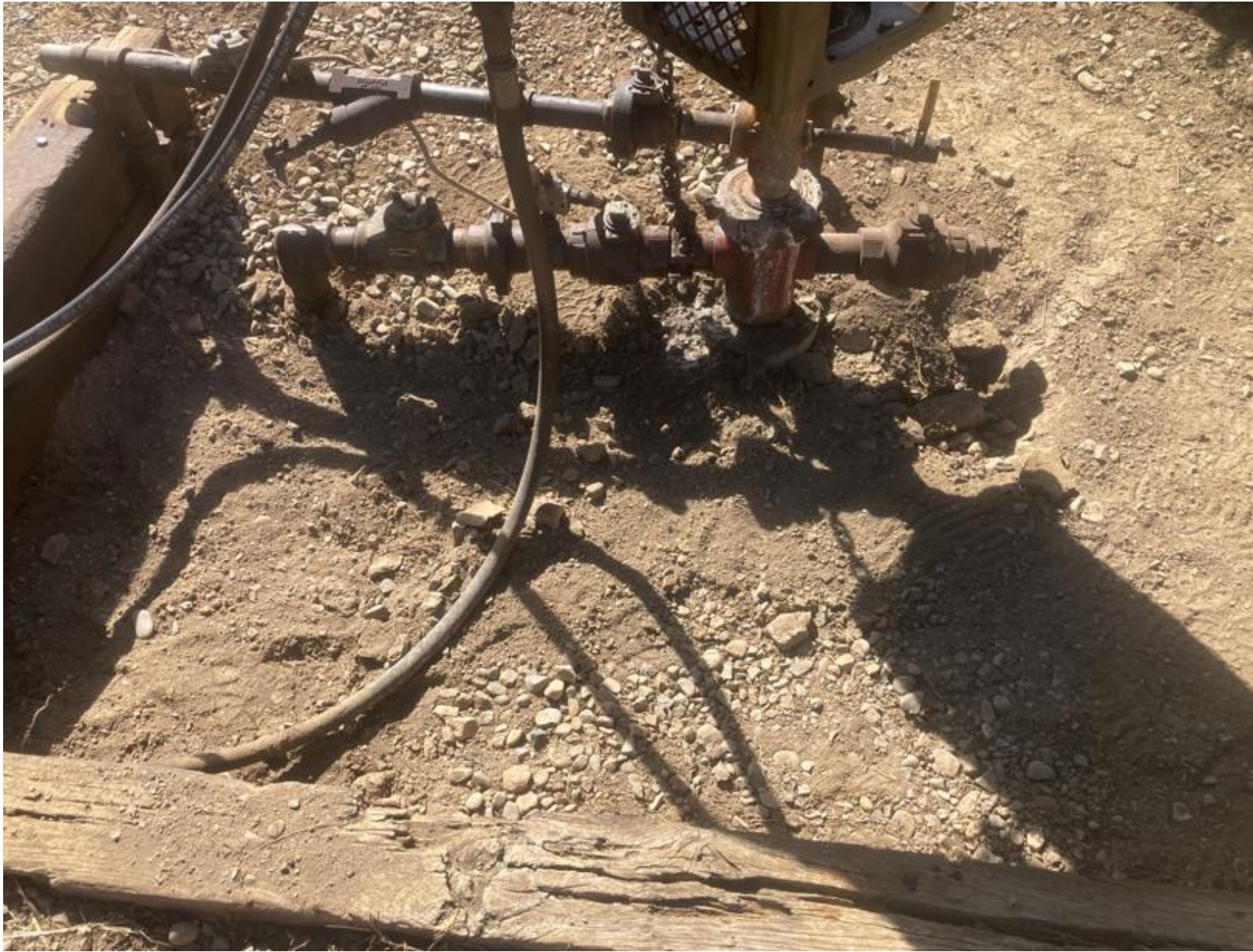
PHOTO 2: THE DRIPPING LEAK HAS BEEN STOPPED AND PACKING ON THE WELL HEAD TIGHTENED. THE IMPACED SOIL HAS BEEN REMOVED FROM AROUND THE WELL HEAD AND FRESH PAD MATERIAL ADDED.
