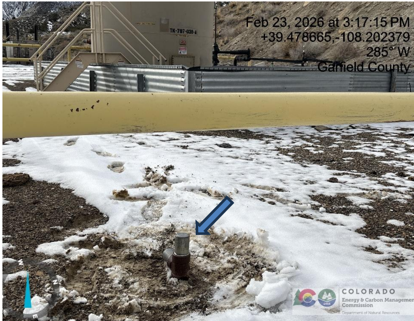
Photo # 2800 Unused flowline lacks lockout tagout (OOSLAT)
