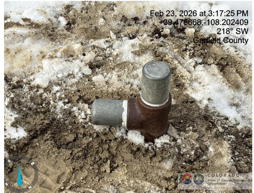
Photo # 2801 Unused flowline lacks lockout tagout (OOSLAT)
