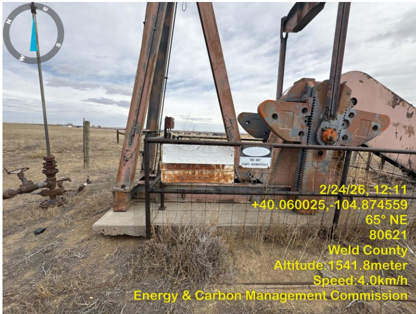
Photo 3 Wellsite sign faded & needs to be updated.
