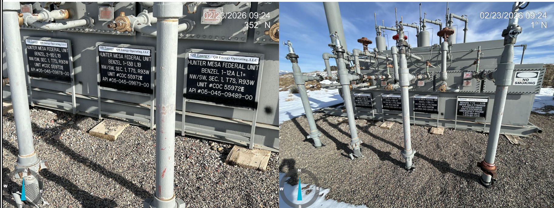
Photo 5: Photos showing some separator signage is missing Emergency Phone Number information; comply with Rule 605.g.
