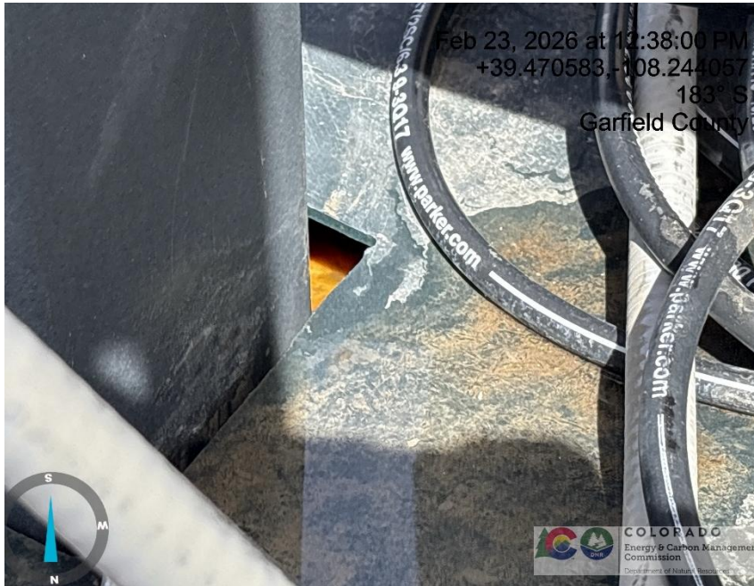
Photo # 2345 Failure to maintain chemical BMP – Chemical tank containment approximately 3/4 full of fluid/BMP not sufficient to contain possible spill
