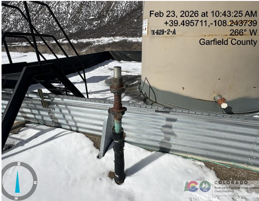
Photo # 1569 Unused flowline lacks lockout tagout (OOSLAT)
