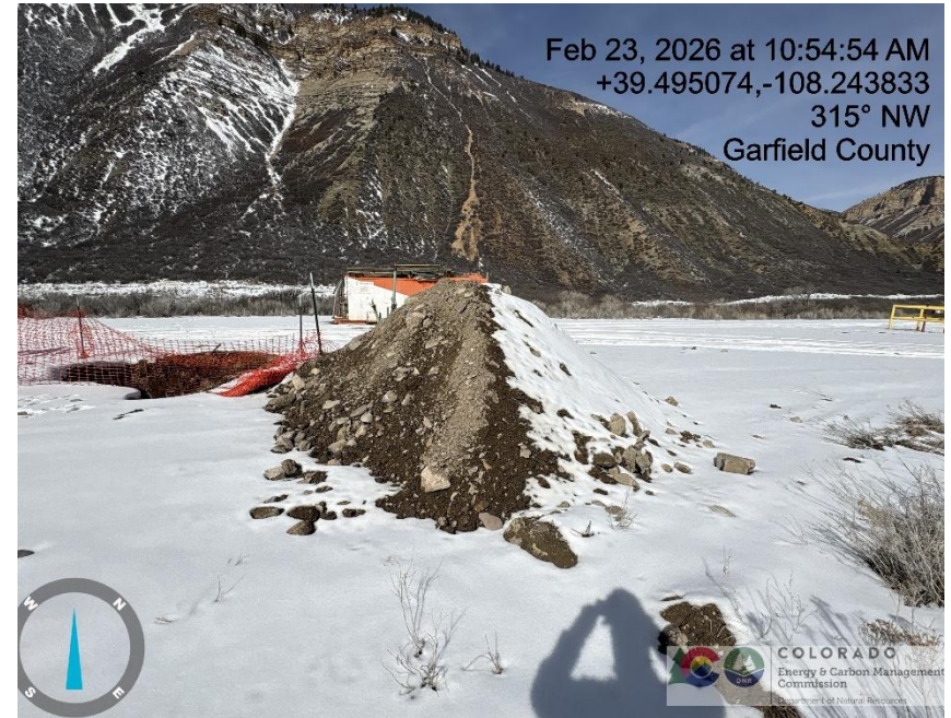
Photo # 1572 Soil stockpile lacks BMP's
