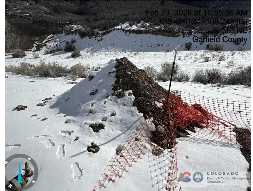
Photo # 1574 Soil stockpile lacks BMP's
