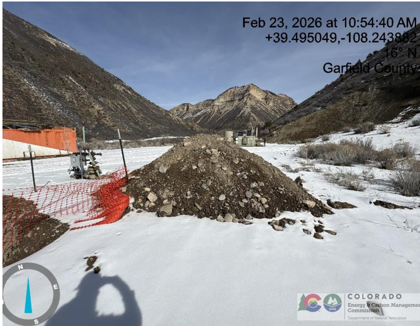
Photo # 1571 Soil stockpile lacks BMP's
